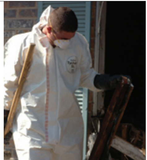
DEMOLITION SGT Marcus Hutto tears out part of a damaged doorway to make it easier to remove items from the house.
