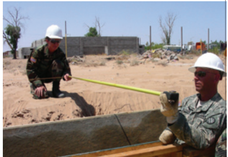
PRECISION SGT Tina Frame and SSG Doug Mecham, both of the 116th Construction Support Equipment Company, UTARNG, ensure the proper distance from the border for concrete footings near San Luis, AZ.
