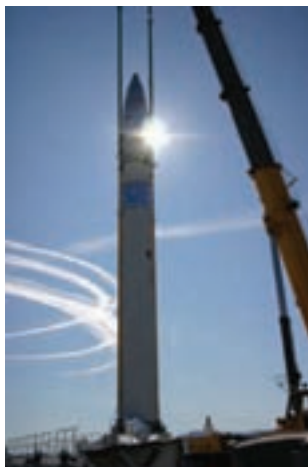
::EMPLACED:: A ground-based interceptor is lowered into its missile silo during a recent emplacement on the Missile Defense Complex at Fort Greely, AK.
