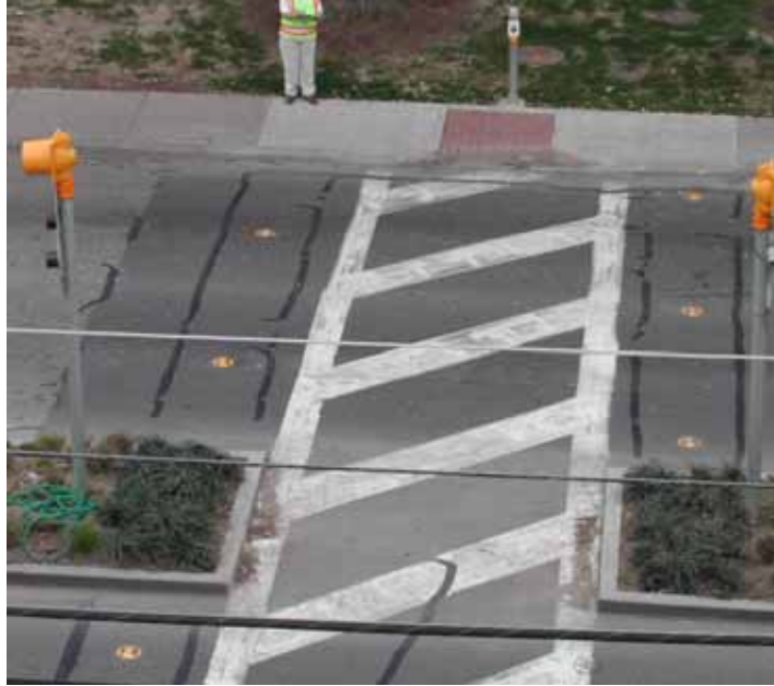
Figure 10-11. Photo. Working example of in-roadway warning lights with pedestrian pushbutton in Austin, Texas.
