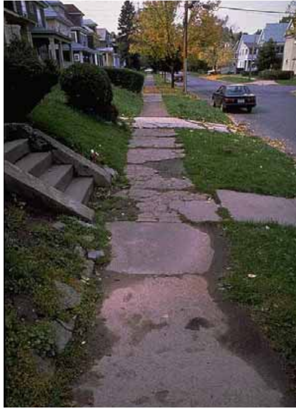
Figure 7-1. Photo. Inadequate maintenance of sidewalks makes a short walk difficult to maneuver.
