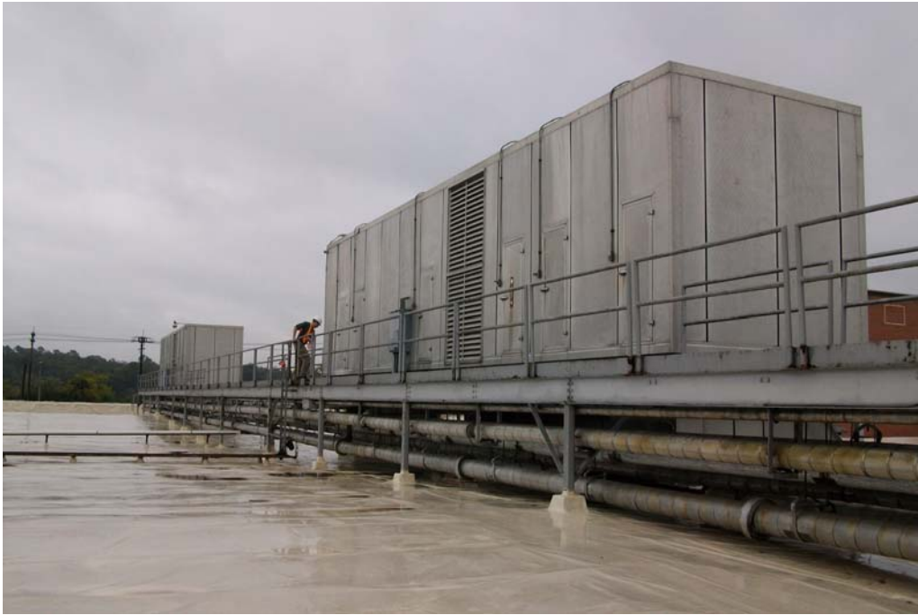
Photograph No. 1: Rooftop air handling units and associated steel support structure above Weave Room No. 2.
