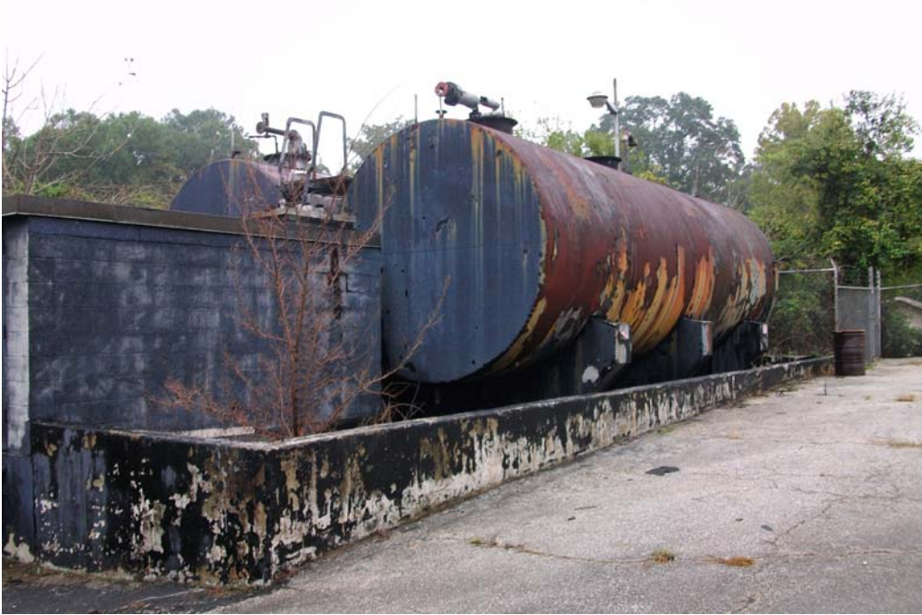
Photograph No. 7: Fuel oil storage tanks.
