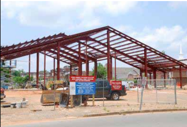
Hattiesburg, MS, May 12, 2009 – Construction crews work on Hattiesburg's fire station. It is one of the few remaining projects in Forrest County's recovery from Hurricane Katrina. Courtesy of Jennifer Smits, FEMA.
