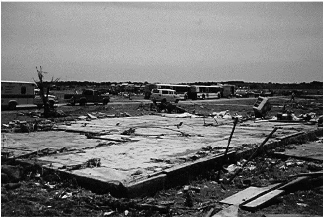
Close-up view of a home foundation in the Double Creek Estates subdivision of Jarrell. Note the plumbing pulled out of the concrete in the center of the picture. Photograph by NWSFO Austin/San Antonio.
