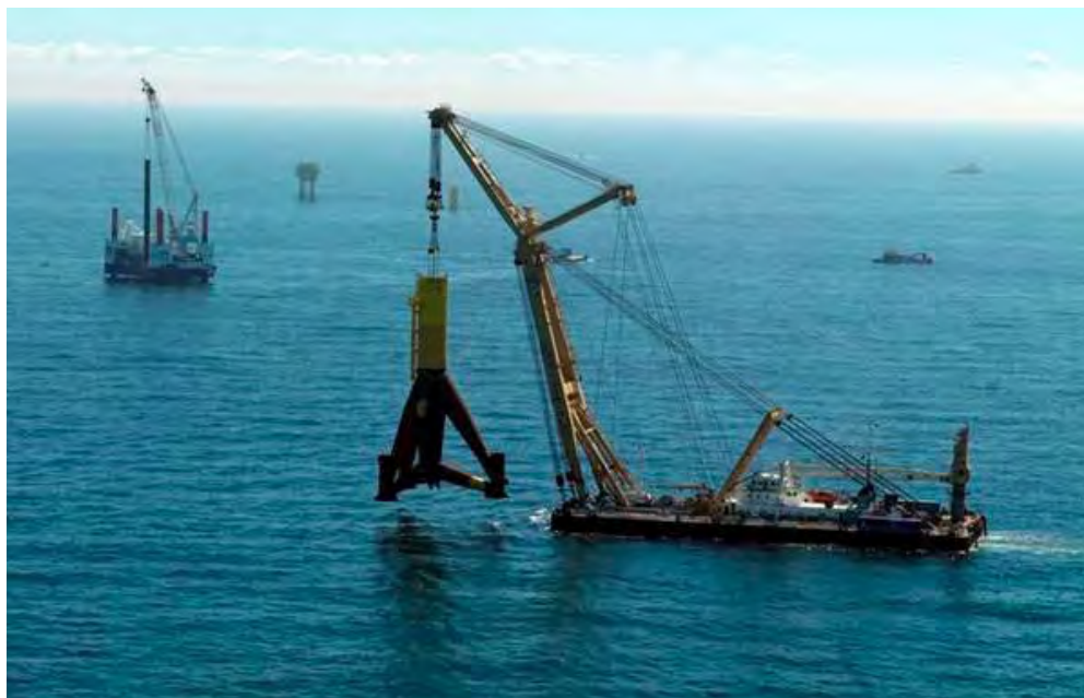
Figure 2.4. The Taklift 4 Placing a Tripod Foundation at Alpha Ventus Source: Alpha Ventus 2010
