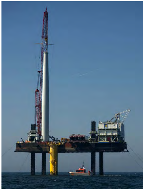
Figure 5.9. Lifting a Fully Assembled Tower onto a Transition Piece at Rhyl Flats Source: RWE npower 2010
