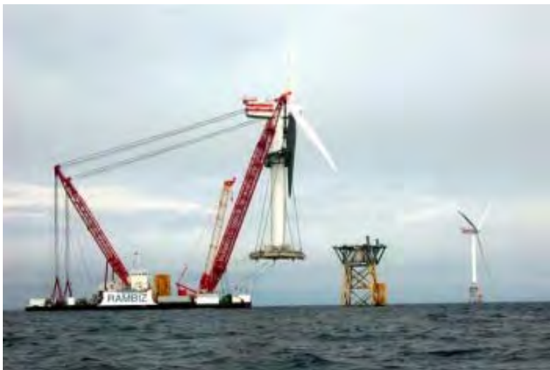
Figure 6.5. The Heavy Lift Vessel Rambiz Installing a Turbine at the Beatrice Project
