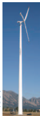
Entegriy EW50 (50 kW) on tubular tower.
