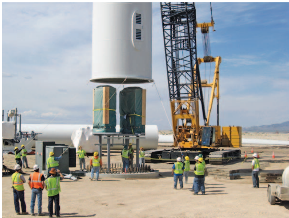
Developer and owner First Wind is constructing a multi-megawatt wind farm in Milford, Utah. Phase I is 145 MW (Clipper turbines) and Phase II is 58.5 MW (GE turbines). Photo credit: First Wind/PIX16738.
