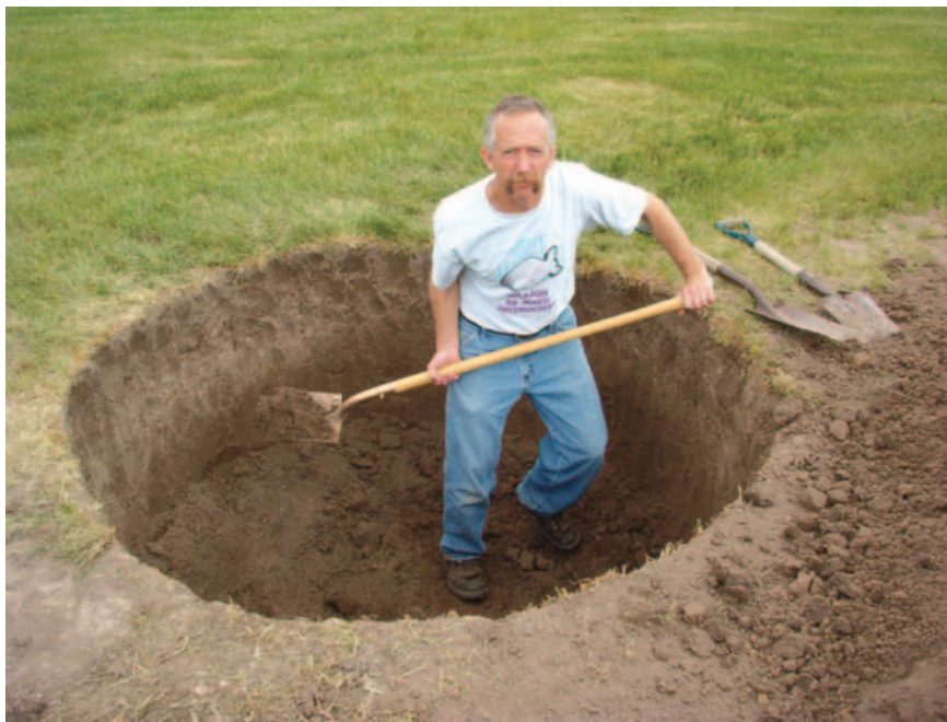
Burlington High School science teacher Jim Jones digs the foundation for the Wind for Schools project turbine. Photo credit: Michael Kostrzewa/PIX16847.
