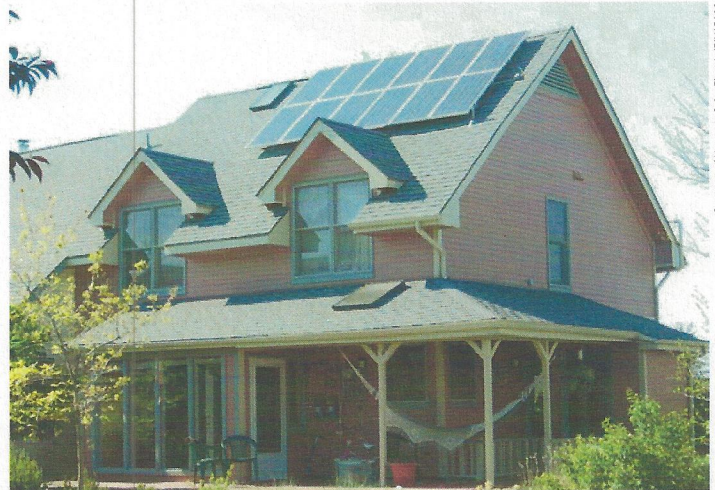
Courtesy of Namaste Solar Electric/PIX16520
