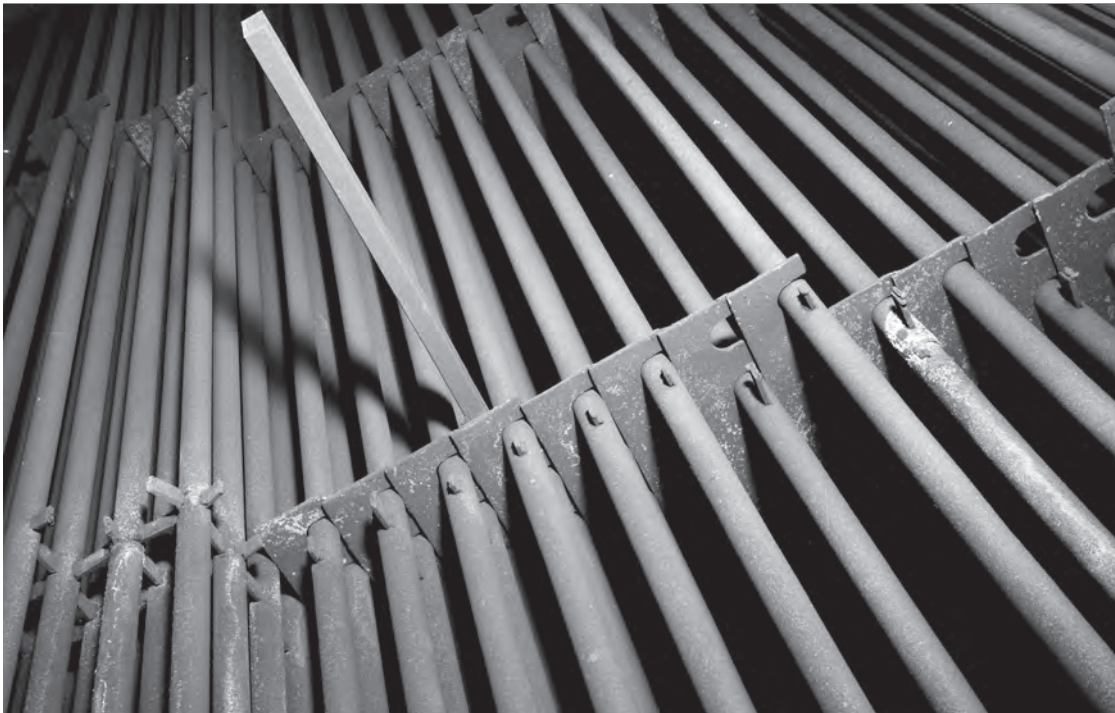
Image 67: Narrow fins or vanes inside the cooler were filled with water. As the 1,000°F to 2,000°F airflow passed between the vanes, heat was transferred from the air to the cooling water. The cooling water was cycled out of the system, carrying with it much of the exhaust heat. This photograph shows the vanes inside PSL No. 2's cooler on 20 January 1959. (NASA C-1959-49583)
