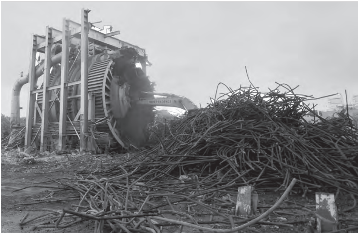
Image 160: Steel cooling vanes from the primary cooler lie in a pile in the foreground on 22 July 2009. A crane tears into the primary cooler in the background. (NASA C-2009-02021)
