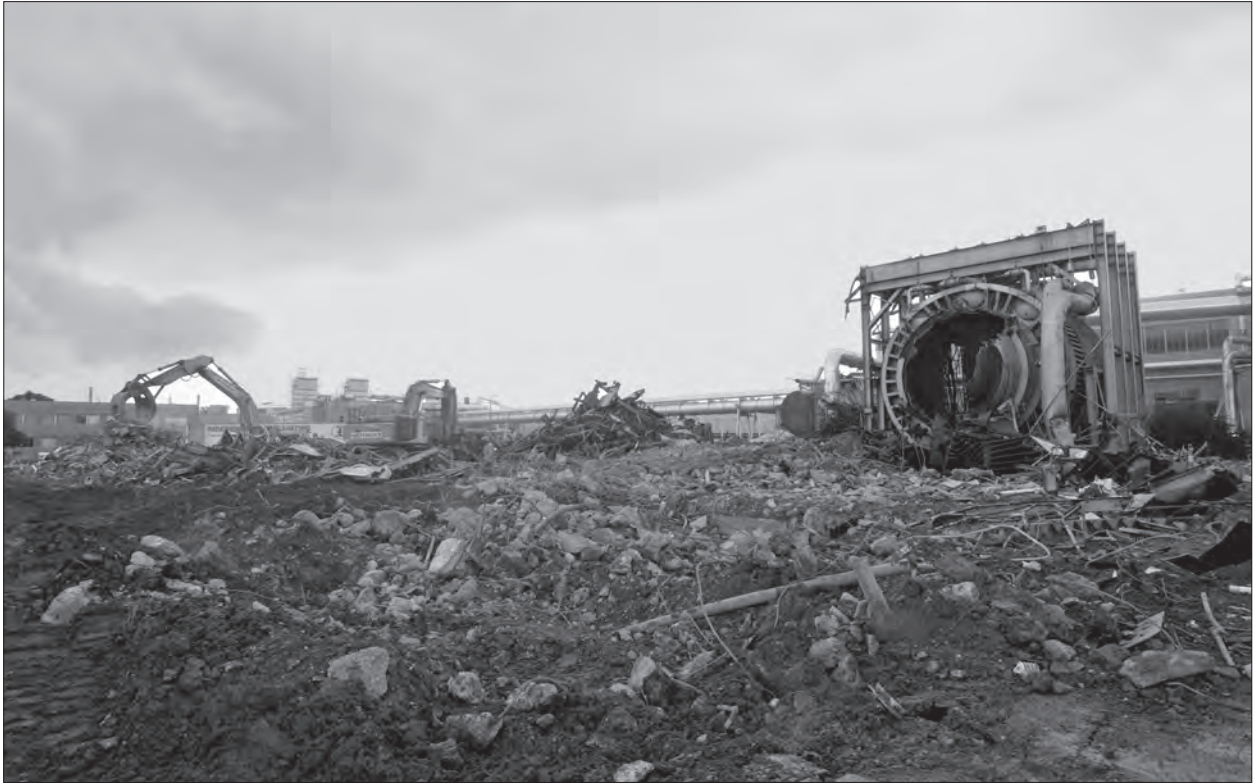
Image 155: PSL wasteland on 1 July 2009. In just over two months, the wrecking crew leveled a facility that had been part of the center's landscape for nearly 60 years. (NASA C-2009-02018)
