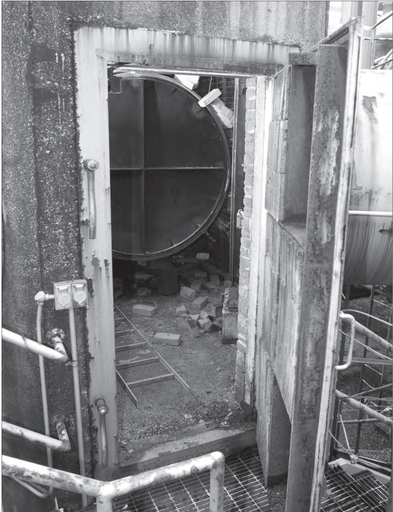
Image 153: Interior of the atmospheric air vent behind the test chambers on 9 September 2008. The facility had been inactive for 30 years. (NASA C-2008-04148)
