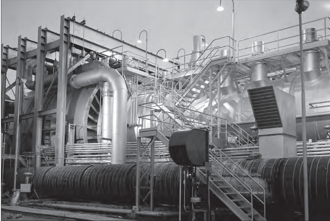
Image 66: Each test chamber had a large primary cooler to reduce the temperature of the extremely hot engine exhaust before the air reached the exhauster equipment. The airflow exited the test section, passed through the chamber's 37-foot-long exhaust section, and then entered the cooler. PSL No. 2's primary cooler is seen here on 24 September 1952. (NASA C-1952-30771)
