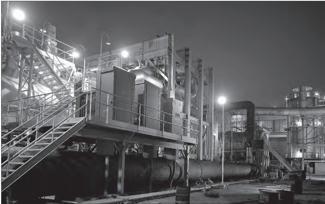
Image 51: "PSL 1 and 2 had lots and lots of pipes and big valves," remembered Howard Wine. "It could take you about an hour just to check the facility out every night prior to running to make sure the valves were all [in the] right sequence....You checked everything, climbed the ladders up to the top, and [made] sure the flow-out disks were all in place and so forth. So it was quite an operation we went through running the facility here." 10 (NASA C-1952-30768)
