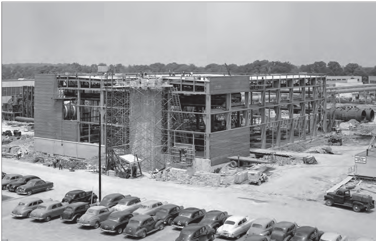
Image 29: Construction of the PSL Equipment Building viewed from the north in July 1951. This structure housed the exhausters and compressors. (NASA C-2009-00166)
