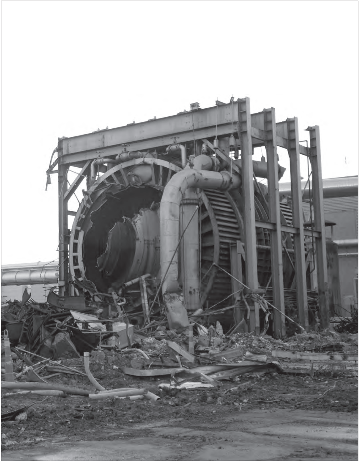
Image 151: NASA Glenn demolished PSL No. 1 and 2 during the summer of 2009. The destruction is nearly complete in this 1 July 2009 photograph. Only one primary cooler remains standing. (C-2009-02016)
