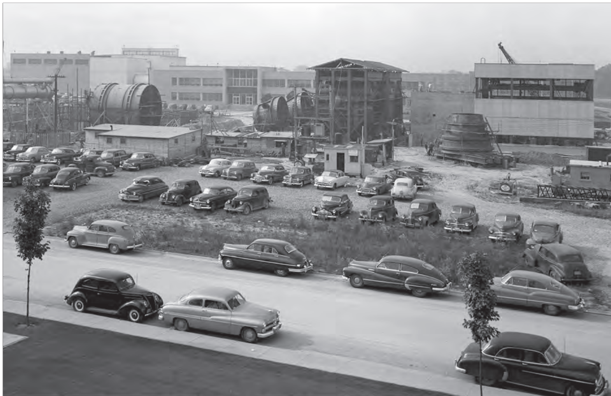
Image 25: This late September 1950 photograph shows the framework for the two primary coolers for the altitude exhaust near the center of the photograph. The Shop and Access Building is being built to the right, and excavation for the Equipment Building has begun in the background to the left. (NASA C-2009-00184)
