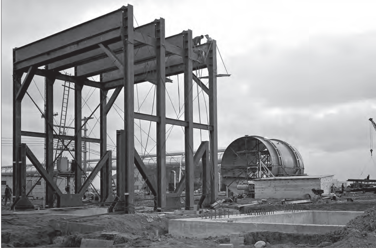
Image 21: Early phases of construction in late December 1949. The steel structure to the left would support one of the large exhaust coolers. The shell of one of the coolers is sitting in the background. By the early spring of 1950, the Shop and Access Building was up, and the massive steel stands for the two primary coolers were in place behind. (NASA C-2009-00151)
