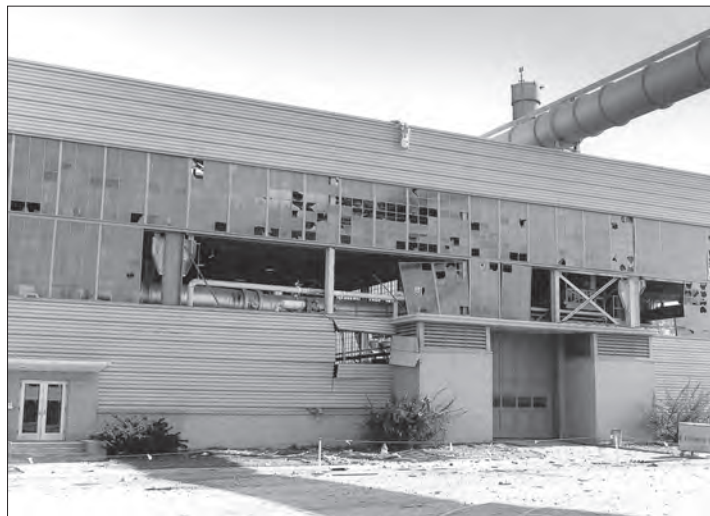
Image 126: An overpressurization in the exhausters in PSL's Equipment Building caused a serious explosion. This 7 April 1971 photograph shows windows blown out on the exterior of the building. (NASA C-1971-01269)
