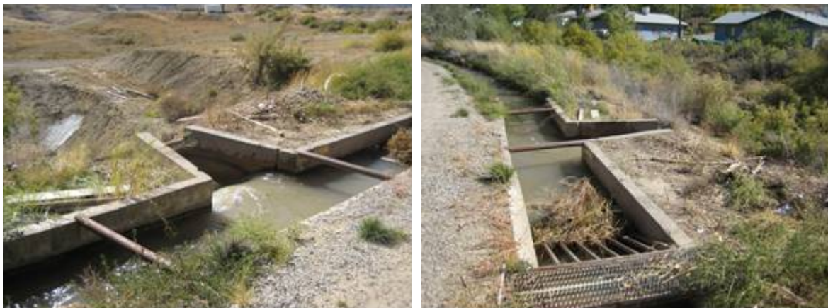
Figure 15. Canal #1 at Rainbow spill. A new flow control structure (fixed orifice) will be installed here to limit the flow into the downstream portion of Canal #1 to its maximum carrying capacity.
