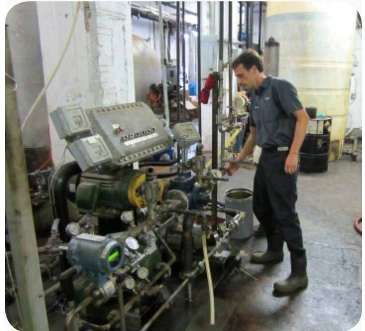
Employee inspecting equipment at Blue Ridge Biofuels, LLC
