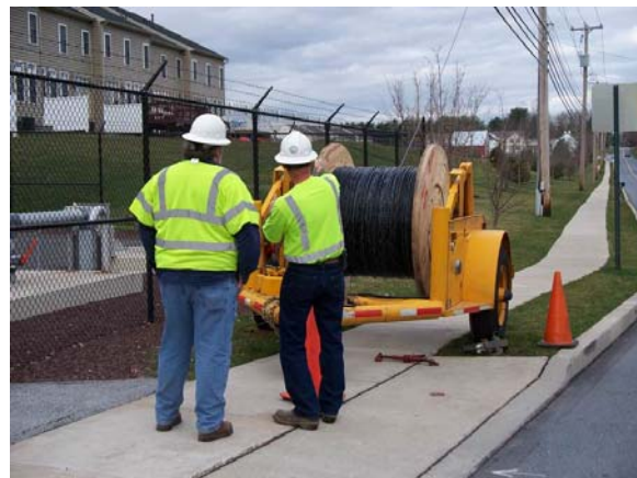
A KINBER crew works with a fiber spool as it prepares to string fiber from poles.
