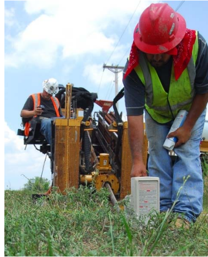
Sho-Me MO contractors use special instruments to carefully locate, measure, and mark directional boring action to place underground fiber conduits.
