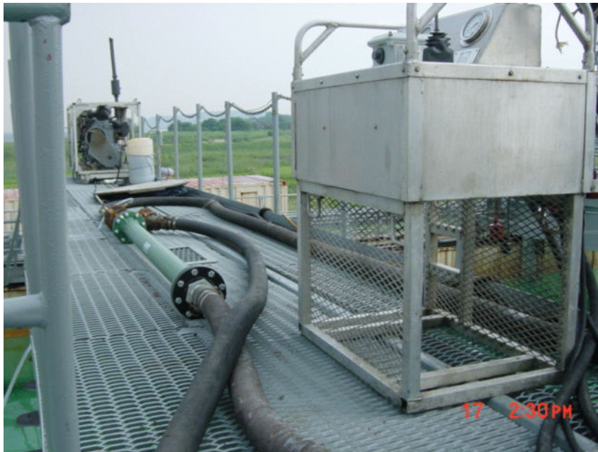
Figure 9. In-line mixer on deck connected to discharge hose just before recovery tanks.
