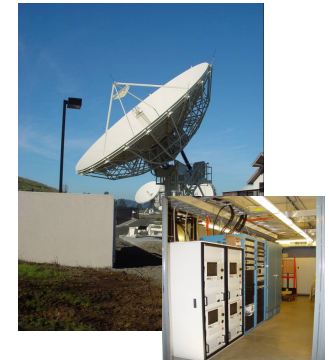
4 Ground Earth Stations
