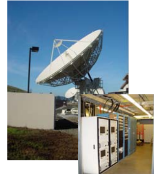
6 Ground Earth Stations
