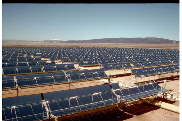
Solar array, California
