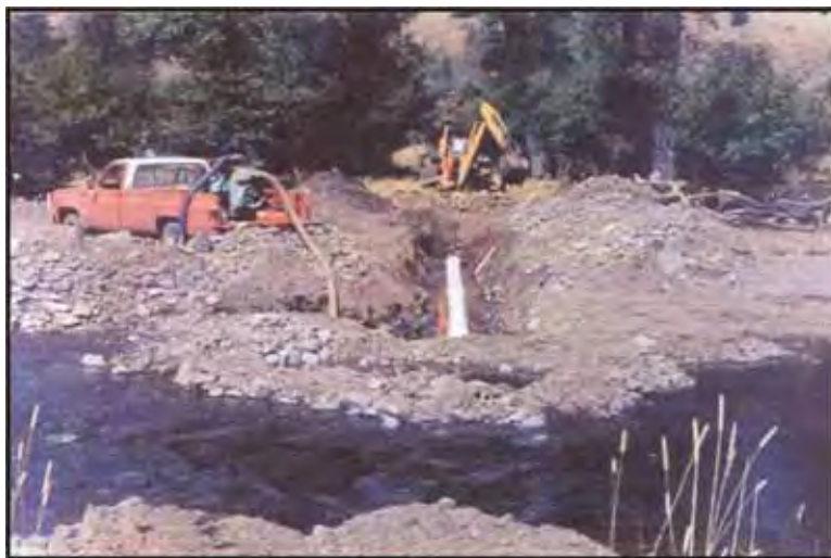
Figure 11. Water delivery pipe feeding lower ditch delivery system from upstream diversion (Holmes pipeline project for USBR).
