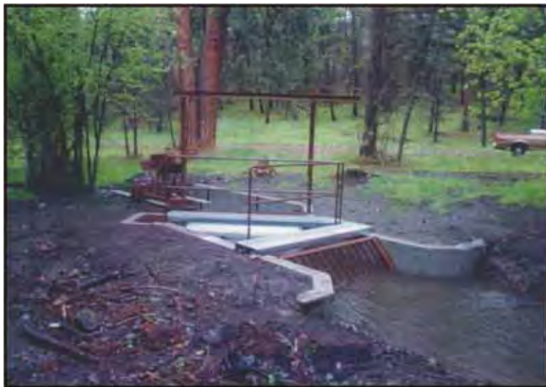
Figure 13b. Single drum fish screen with trash rack.
