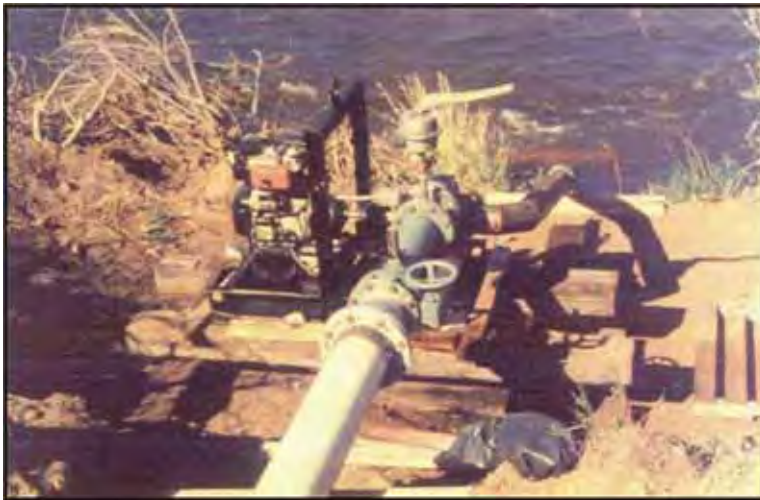
Figure 9. Pump at permanent pump station (1994 Cathedral Rock ditches project for USBR).
