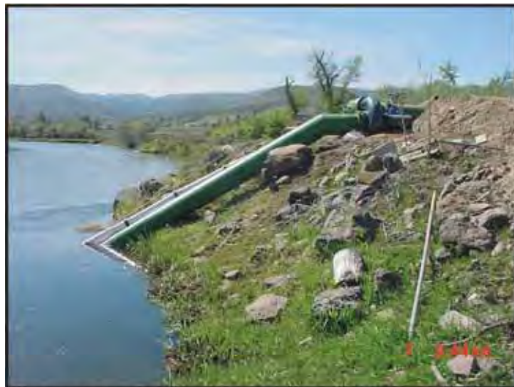
Figure 10. Intake pipe at permanent pump station.
