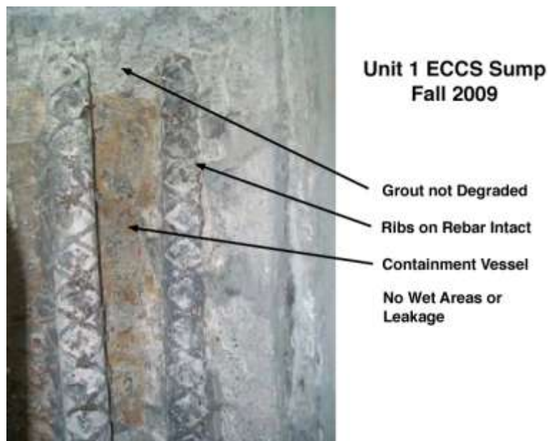
Figure A.6-5 Condition of containment shell, grout, and concrete steel reinforcement in Unit 1 ECCS after grout removal
