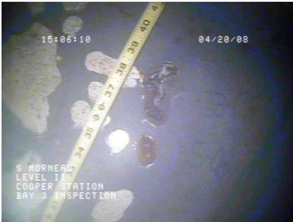
Figure C.1-1 Example of pitting corrosion in torus
