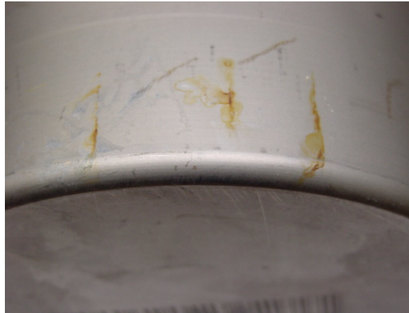
Figure 38 ThroughWall Stress Corrosion Cracks in a Welded Stainless Steel Container not Subjected to Applied Stresses [SRNL Micrograph].
