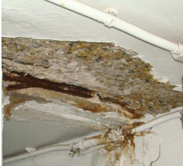
Figure 50 Spallation of Concrete Induced by Rebar Corrosion [SRNL Photograph].
