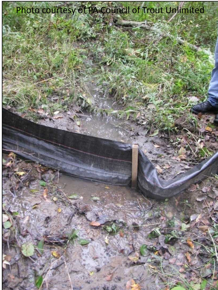
Outlets of sediment control structures are NOT stabilized
