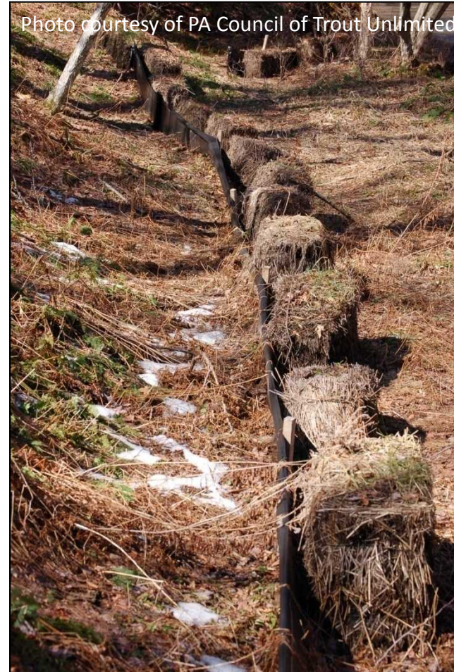
Outlets of sediment control structures are stabilized
