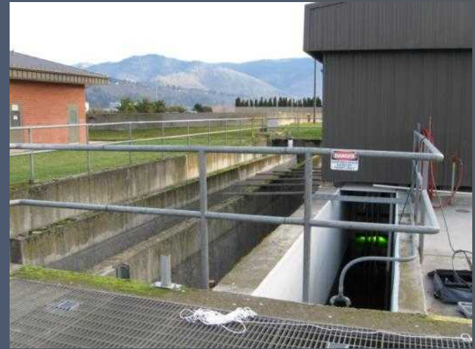
Hood River Wastewater Treatment Plant
