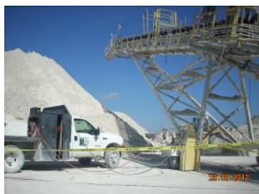
Victim was bolting a snub pulley in position when he fell 16 feet from an elevated walkway to the ground below.
