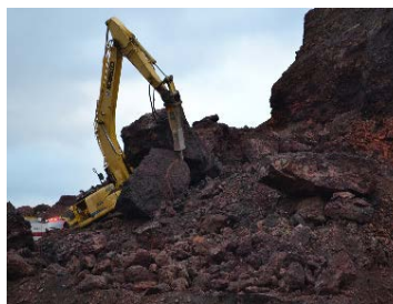
Victim was operating an excavator with a rock breaker when the face of a vertical wall fell onto the cab.
