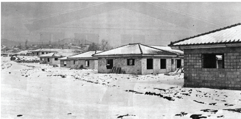
Family housing under construction for the office of the Economic Coordinator, Seoul
