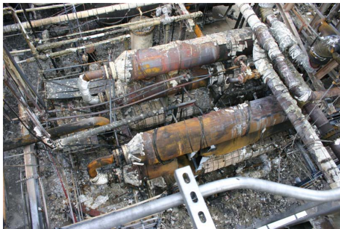
Figure 1: Aerial view of the damaged heat exchangers following the April 2, 2010 fire
