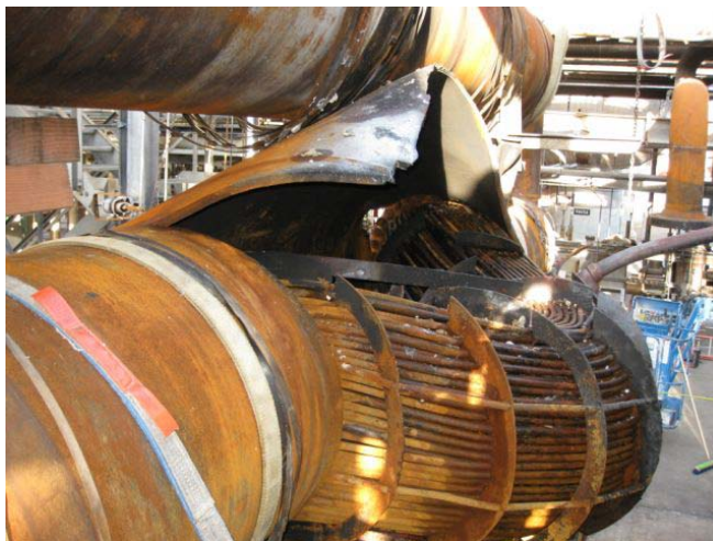
Figure 2: Close-up of ruptured heat exchanger
