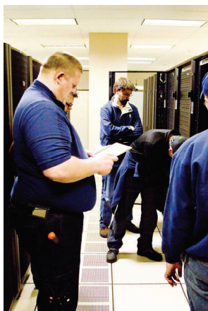
Campus C move, installing servers in the SLDC
