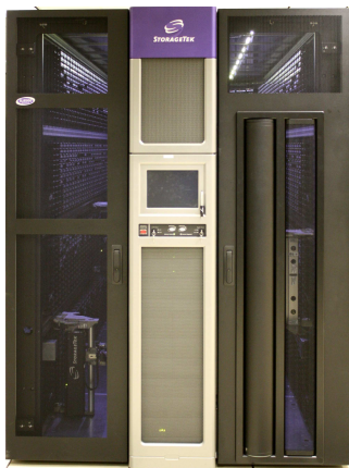
StorageTek Backup Tape Library
