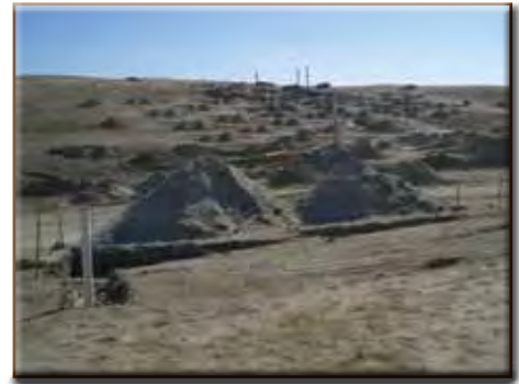
Cameco Resources Smith Ranch Mine during installation of ISR wellfield Converse County, Wyoming
