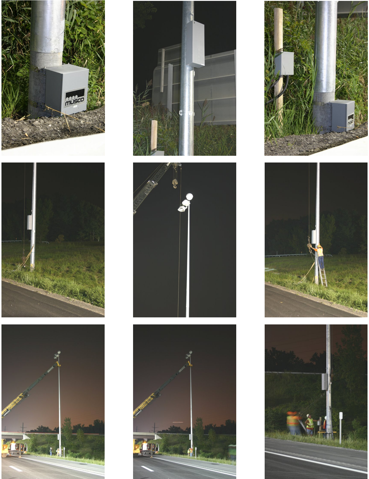
Figure A-2.4. Detail of the control boxes mounted to the poles and sequence during removal of the poles. See Figure A-2.5 for the rest of the removal steps. [Photo credits: Dennis Guyon, Lighting Research Center]
