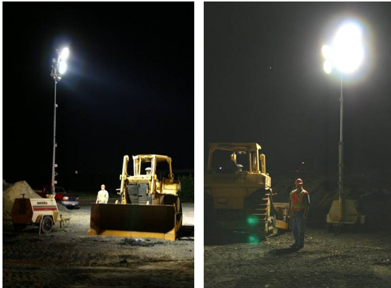
Figure 12. Example of the light and dark zones that are created with typical light towers in a work zone.
