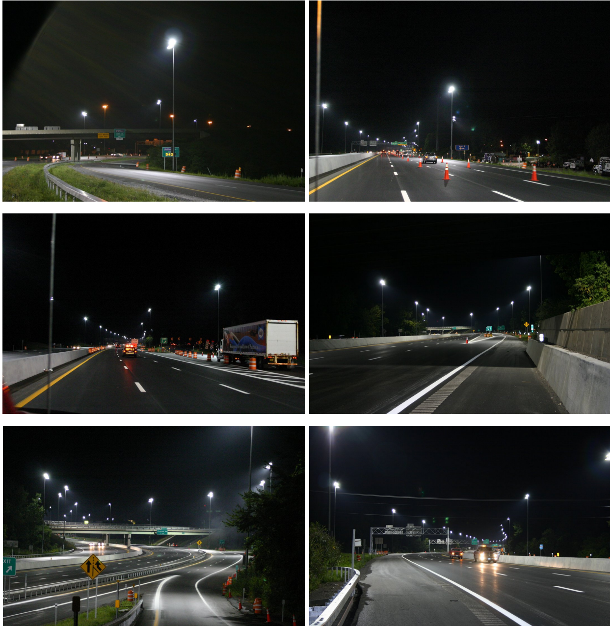
Figure A-2.1. Different general views of the I-90 stretch under construction as it was illuminated with a semi-permanent high-mast lighting system. [Photo credits: Dennis Guyon, Lighting Research Center]
