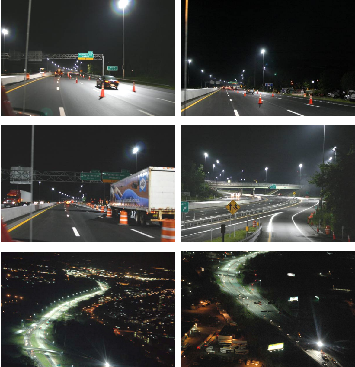
Figure 1. Different views of the semi-permanent high-mast lighting installation on I-90 between Exit 5 and the New York Thruway. [Photo credits: Top and middle rows, Dennis Guyon-LRC; bottom row, MUSCO Lighting.]
