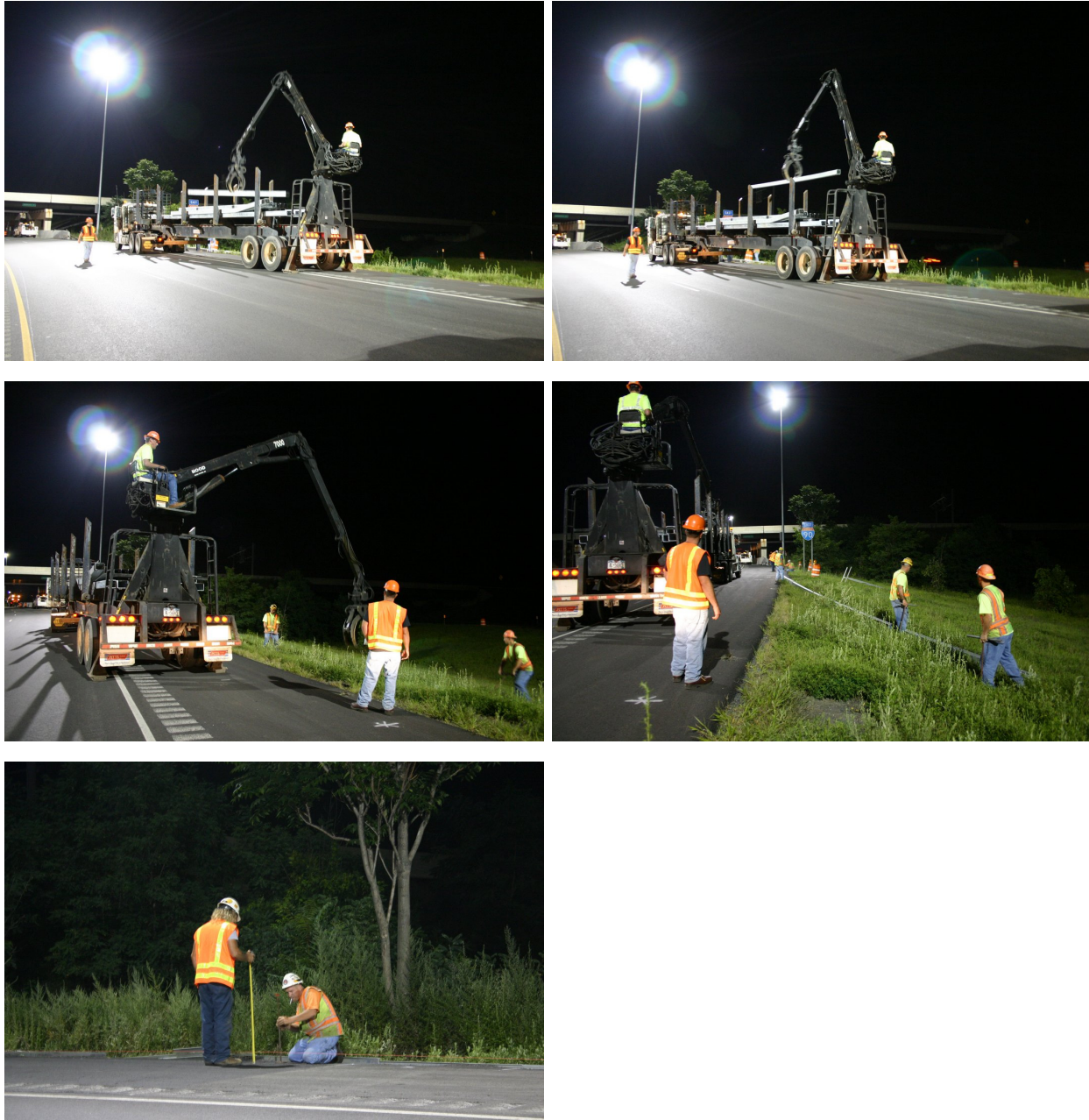
Figure A-2.3. Crew working on the installation of guard rails. It can be appreciated in the photographs the high light levels and uniformity provided by the lighting and how the coverage beyond the clear zone was also helpful with some of the maintenance tasks. [Photo credits: Dennis Guyon, Lighting Research Center]
