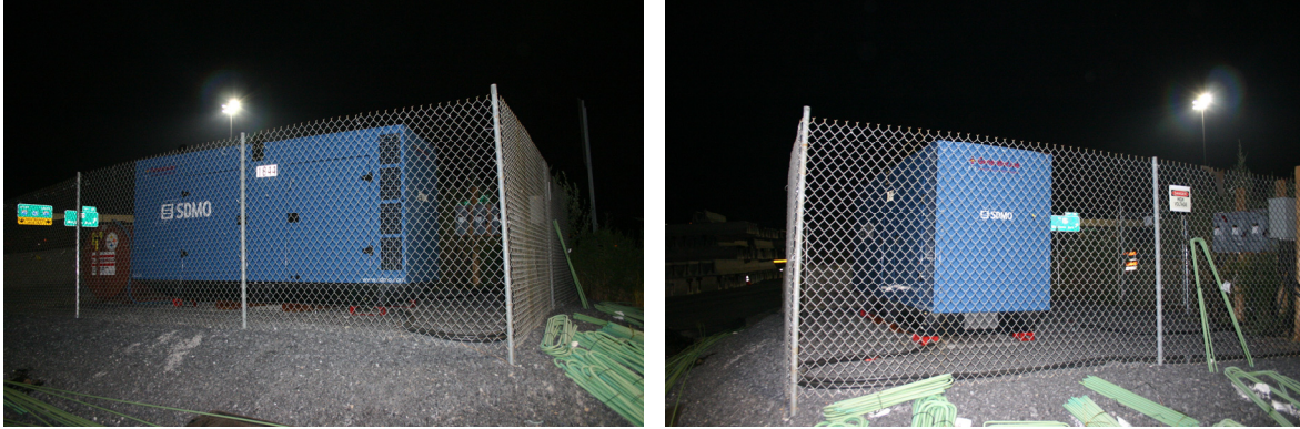
Figure A-1.1. Photographs of generator #1 (Gen #1) located on the contractors yard near Exit 2.
