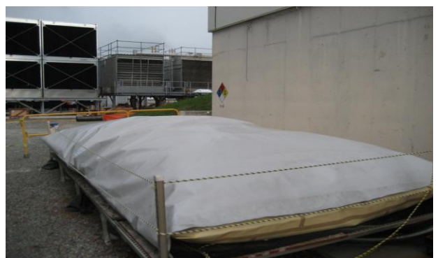
GTS SF6 Storage (building exterior / filled)
