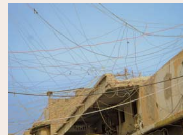
Makeshift distribution wires from private generators
