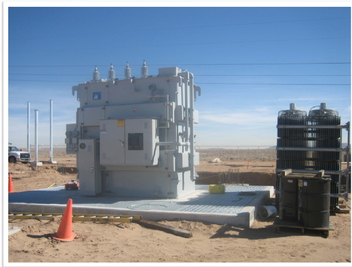
Navajo Tribal Utility Authority – substation
