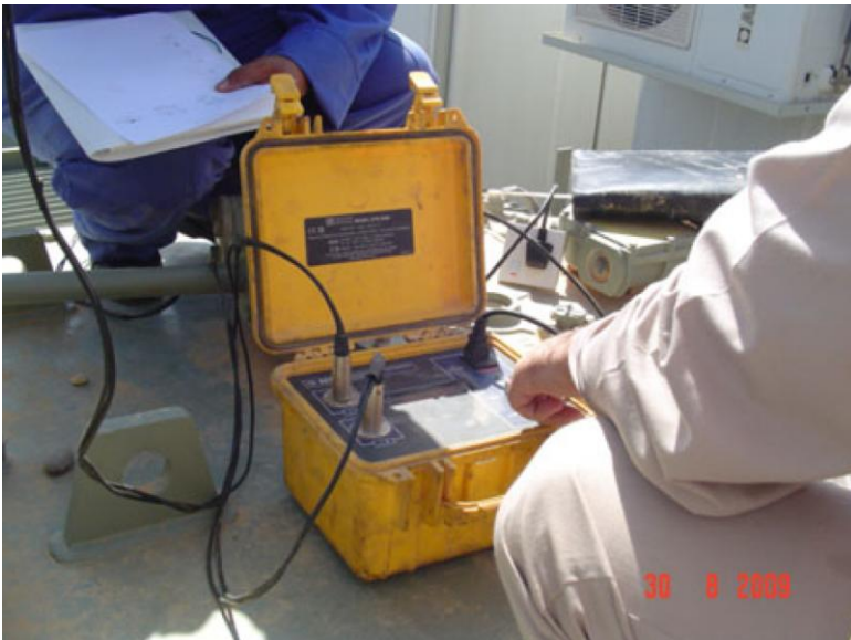
Site Photo 4. Testing of mobile substations after delivery (Courtesy of GRC)
