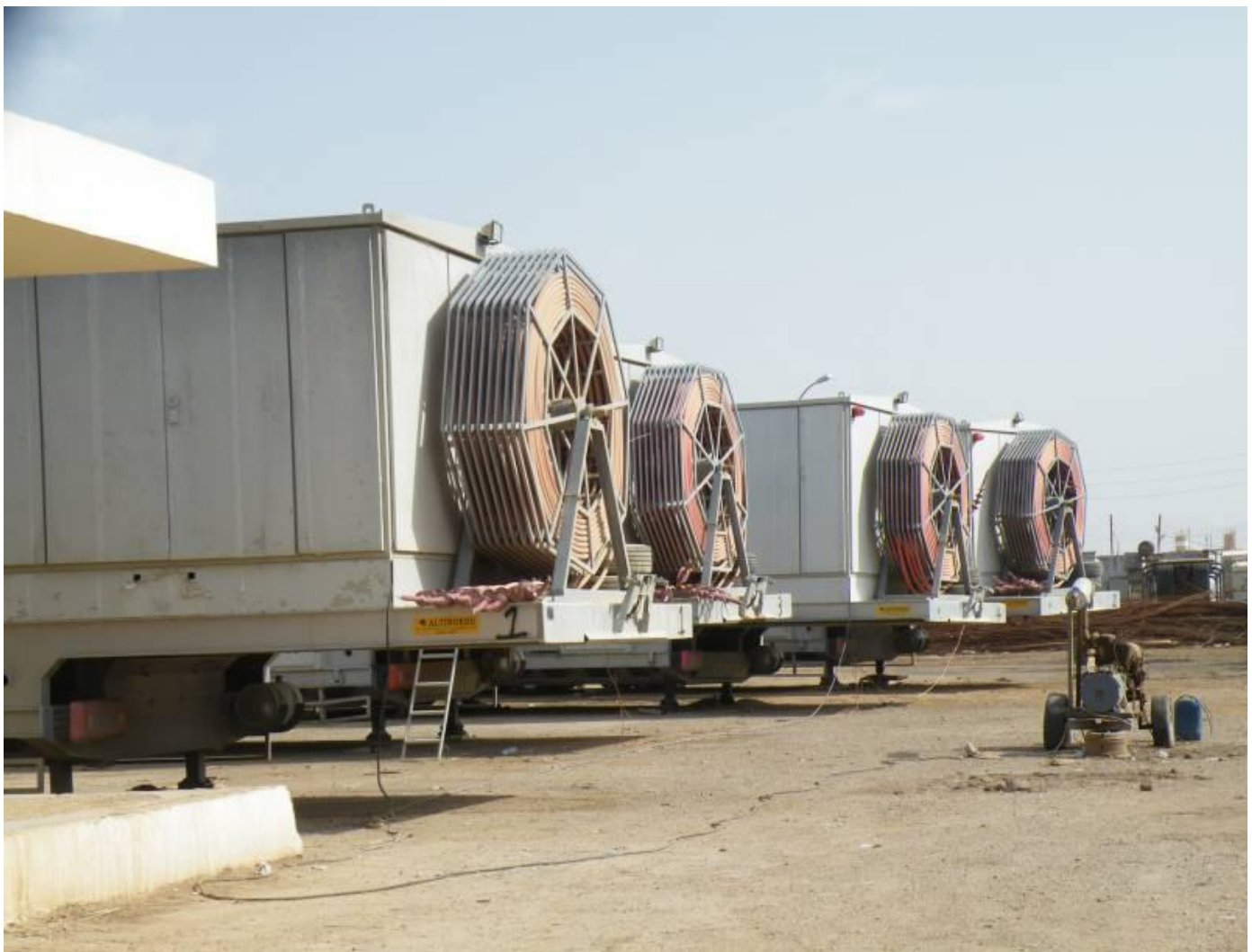
Site Photo 6. Four mobile electrical substations at the MOE's Ramadi outdoor warehouse facility
