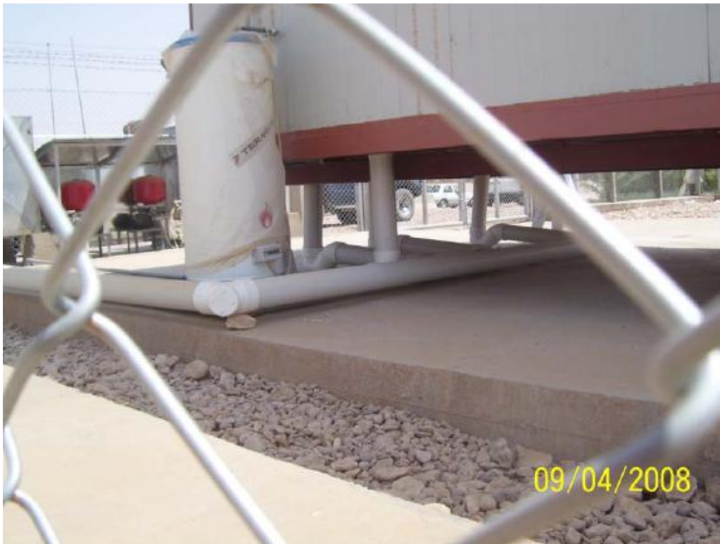
Site Photo 3. A rock used to improperly pitch the sanitary line (Courtesy of GRC)
