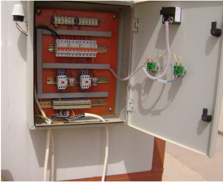
Site Photo 1. Cables unsecure and not in conduit (Courtesy of GRC)
