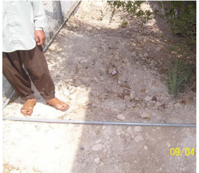
Site Photo 2. Water supply to guard house not buried (Courtesy of GRC)
