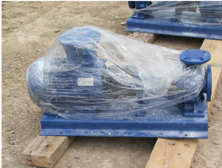
Site Photo 14. Pumps for fuel oil transfer
