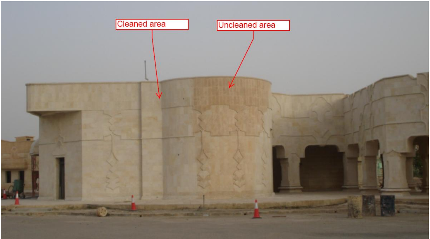
Site Photo 1. Example of renovation work – cleaning of the exterior building (Courtesy of USACE)
