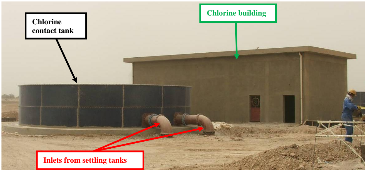
Site Photo 13. Chlorine contact tank and chlorine building
