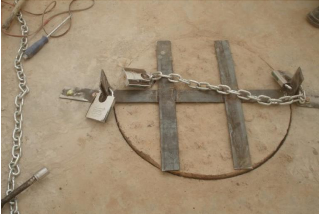
Site Photo 3. Force Main manhole locked by contractor over non-payment of DFI contract (Photo courtesy of the USACE)
