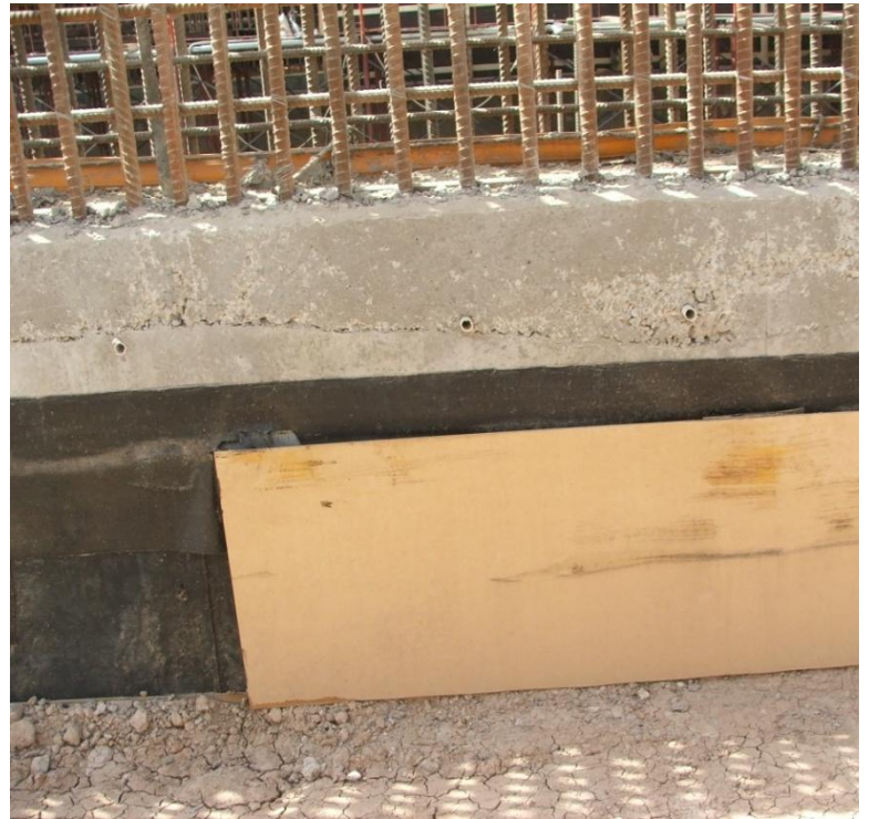
Site Photo 21. Inadequate concrete area (behind cover)
