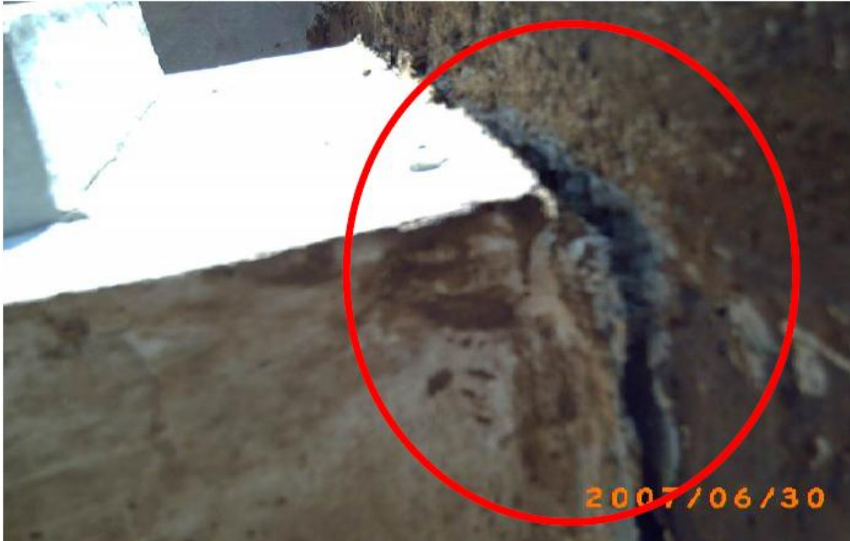
Site Photo 22. Deficiency identified in daily QA report by field engineers (Courtesy of the USACE)
