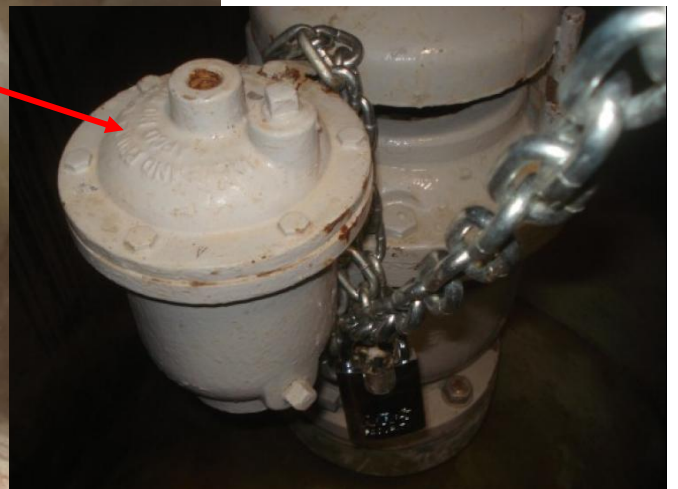
Site Photo 5. Close up of Site Photo 4
