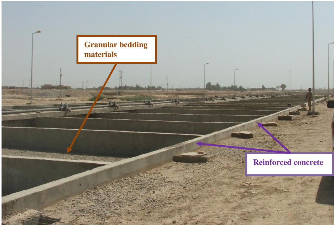
Site Photo 17. Sludge drying beds
