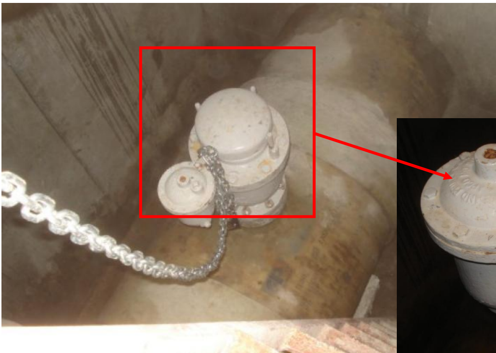
Site Photo 4. Force Main valve box locked by contractor (Photos courtesy of the USACE)
