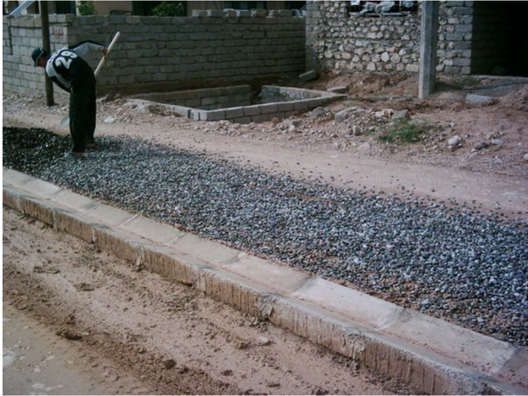
Site Photo 2. Road excavation, leveling, and rolling of the sub-grade (Photo courtesy of USACE)
