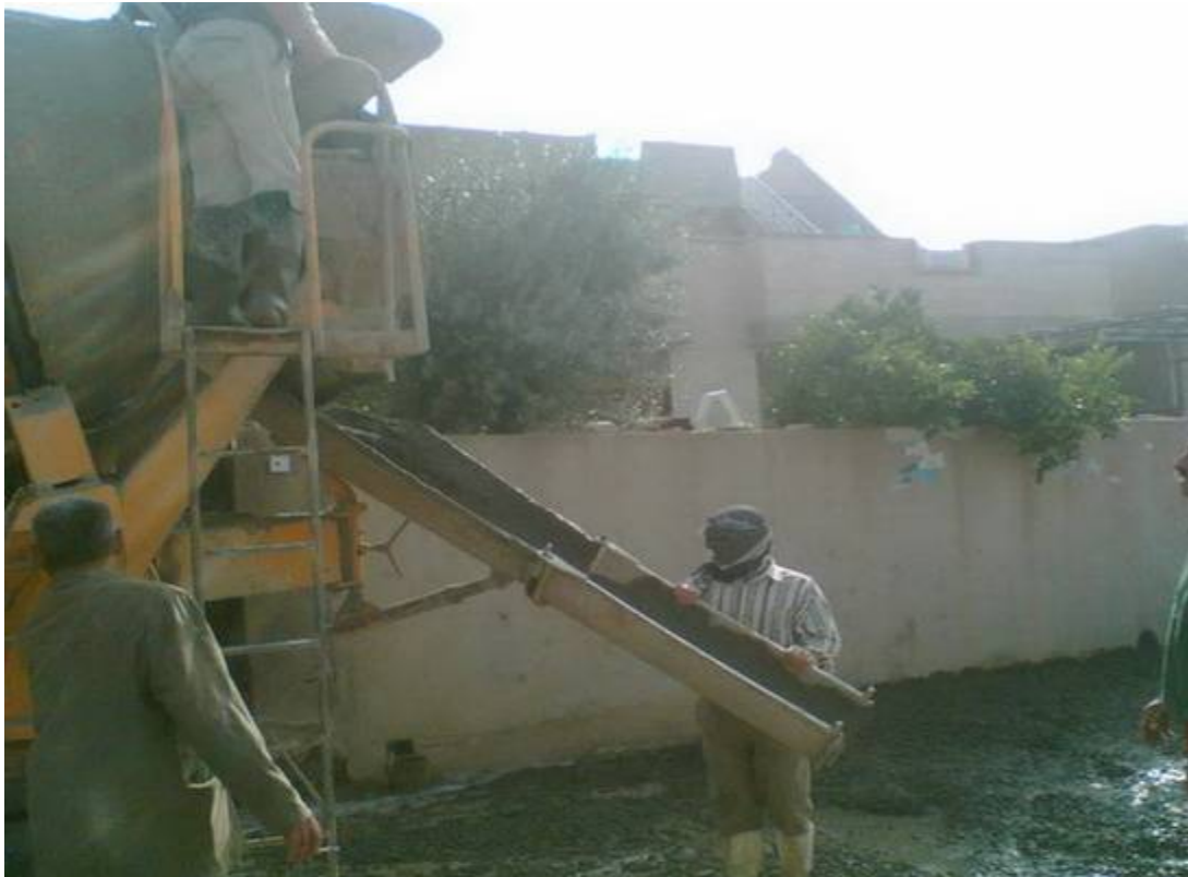
Site Photo 3. Aggregate base and concrete base pour (Photo courtesy of USACE)
