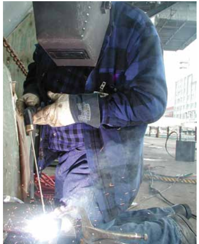
Bremerton, WA (Jun. 8, 2002) Wayne Weight, a shipyard worker from Paulsbo, WA, works on revamping the JP-5 fuel-overflow system on the aircraft carrier USS Carl Vinson (CVN 70). Carl Vinson is eliminating 34 of its 52 JP-5 fuel-overflow boxes and installing a more efficient pipe system. The remaining 18 overflow boxes are being replaced following an extensive deployment in support of Operation Enduring Freedom. (U.S. Navy photo by Photographer's Mate Airman Ryan Jackson)
