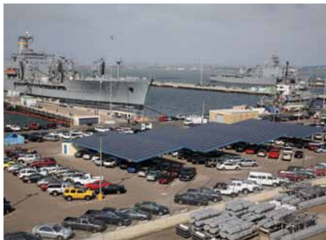
SAN DIEGO, CA Solar photovoltaic power systems (SPVPS) installed at Naval Base San Diego (NBSD) are utilized to generate alternative energy to supply power to the base's buildings.
