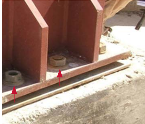
Example where one foundation bolt extends beyond the nut and another bolt does not.
