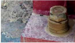
Poor installation technique (use of seven washers).
