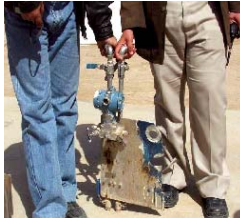
The disabled flow meter for the high-service pump station meter vault.
