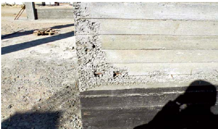
Unacceptable cement pour with honeycombing and exposed rebar at the Missan Surgical Hospital.
