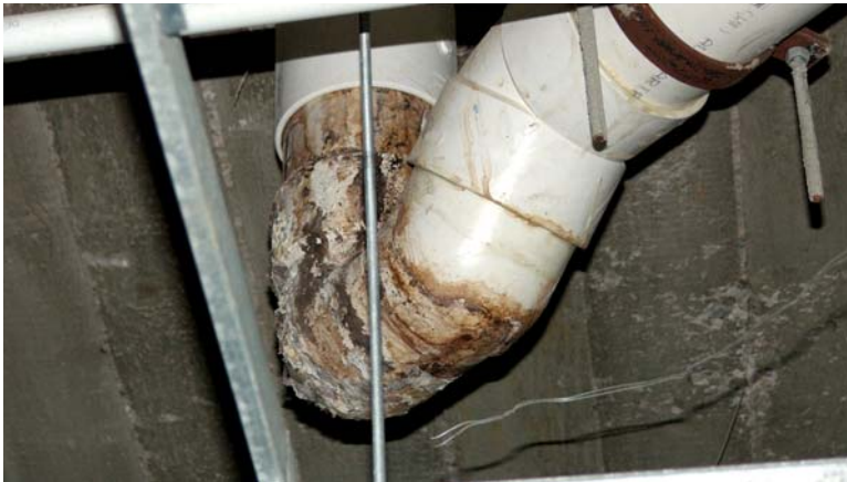
Effluent leaking from pipes at the newly constructed Baghdad Police College.
