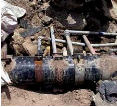
Illegal taps in the transmission and distribution lines, which reduce the water pressure and amount of water available to residents. (USAID photo)
