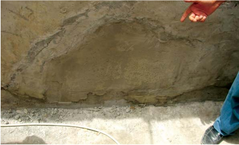
Unacceptable cement pour at a Falluja Waste Water Treatment System pump station.
