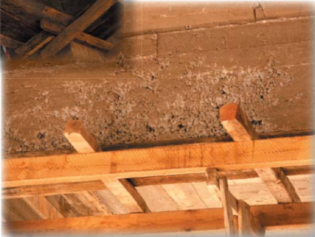
Structural overhead beam with honeycombing and metal reinforcement visible.
