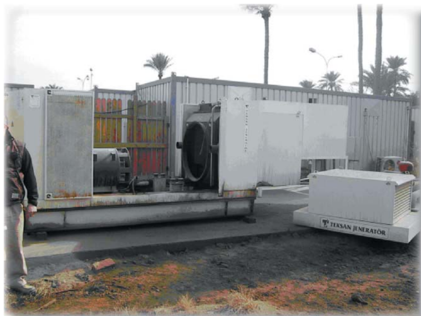
Shell for the 500-kilowatt generator undergoing repairs at the Babylon Police Academy.
