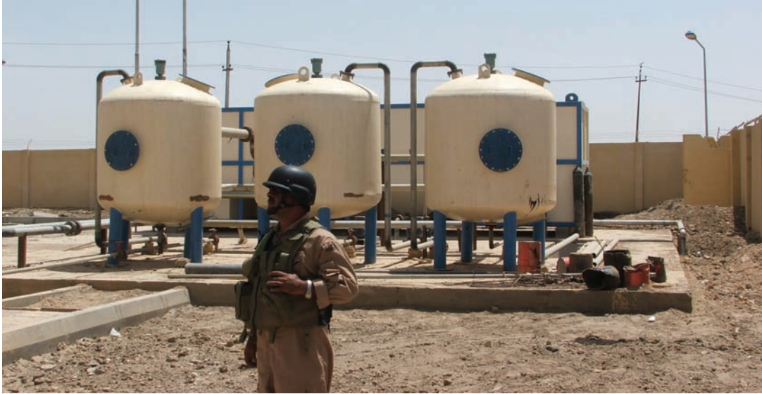
Water compact unit without sunshade at Al Kazim.
