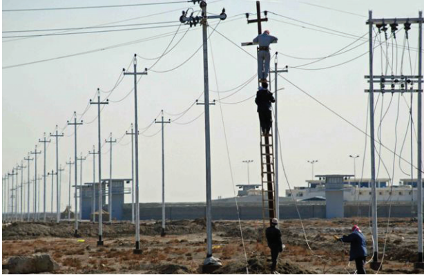
Electricians energize power to Electrical Overhead Feeder of Nassriya Prison. (USACE photo)
