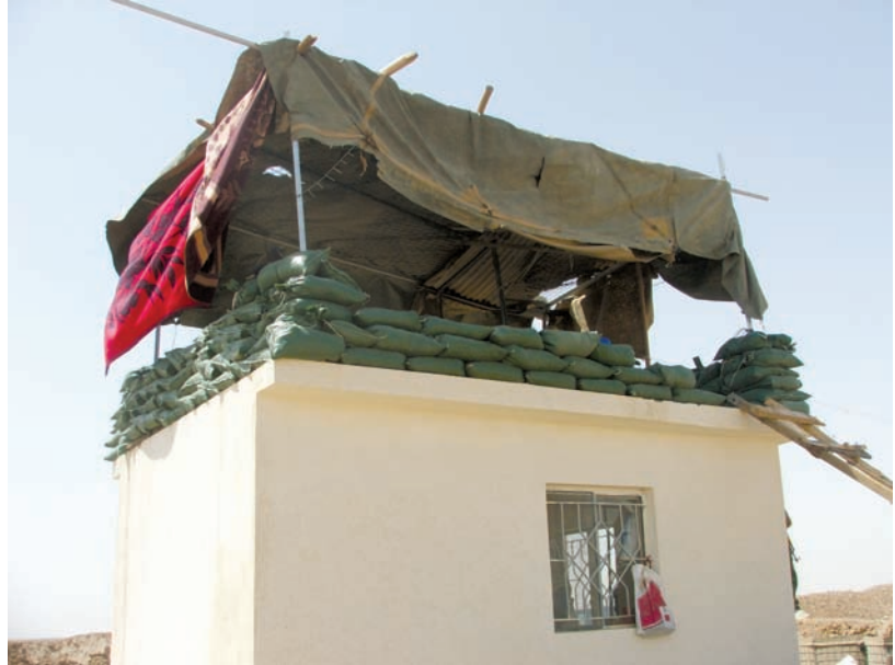
Guard tower constructed by Iraqi Army on roof of guard house, part of the PEZ project.
