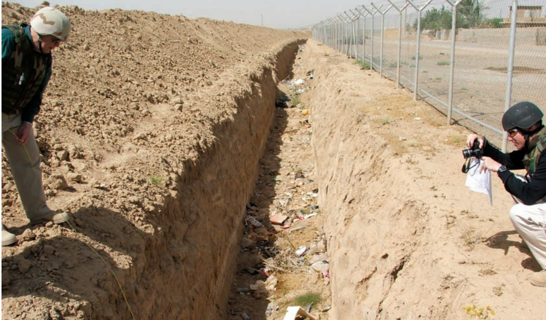
SIGIR inspectors ensuring that the ditch and berm met contract design specifications on the PEZ project.
