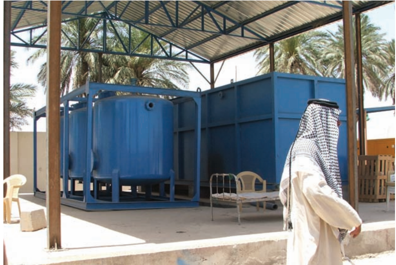
Water compact unit with sunshade at Al Shofa.
