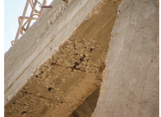
Example of exposed rebar and severe concrete segregation and honeycombing at Kahn Bani Sa'ad.
