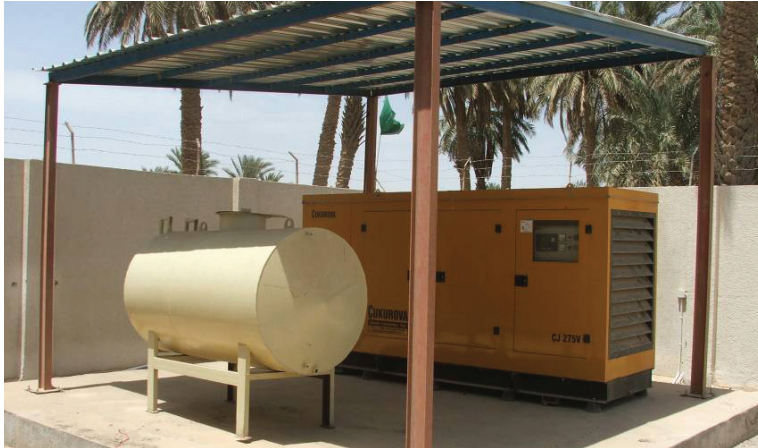
Sunshade for the generator and the fuel tank at Al Shofa.
