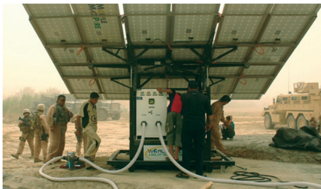
Solar-powered pump provides drinking water for Iraqis in Falluja. (U.S. Embassy photo)
