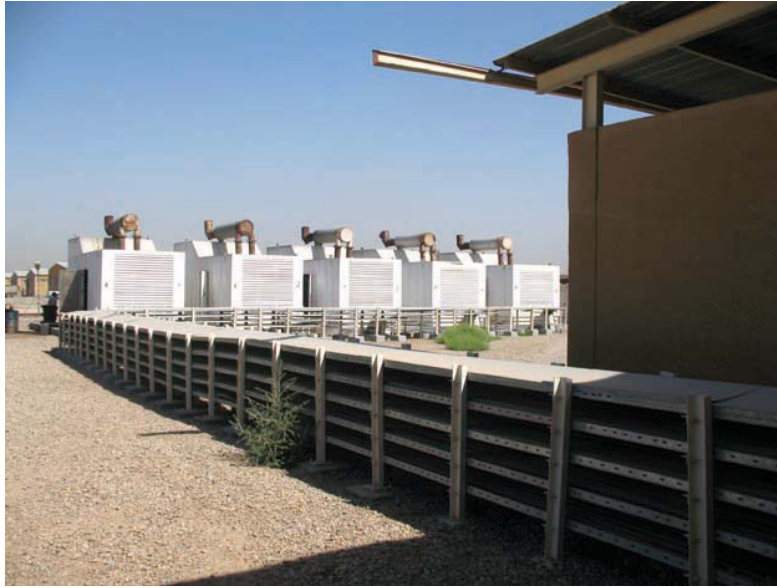
Generators and cable trays running to the electrical room.
