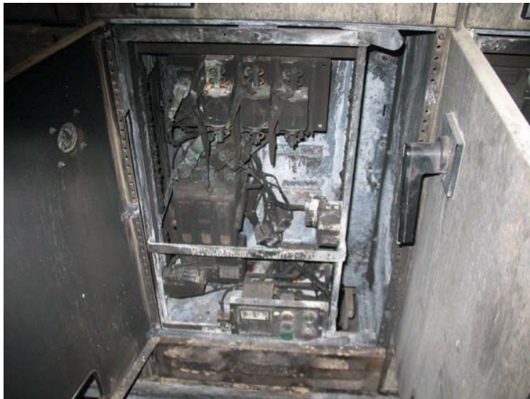
Burnt wiring in the control center at the Doura Power Station. The fire resulted from exciter flashover caused by repeated "hard tripping."
