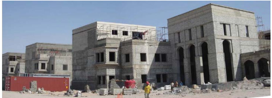
Basrah Children's Hospital. Construction is now scheduled to be completed in July 2008.
