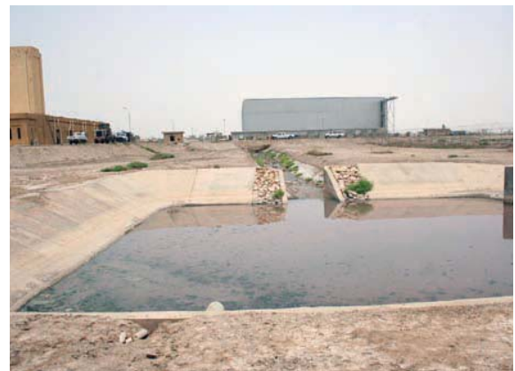
Storm drainage collection pond containing raw sewage.
