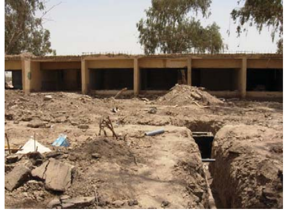
Pre-construction state of building B-230 front view. Extensive renovation work needed (contractor-provided photo).
