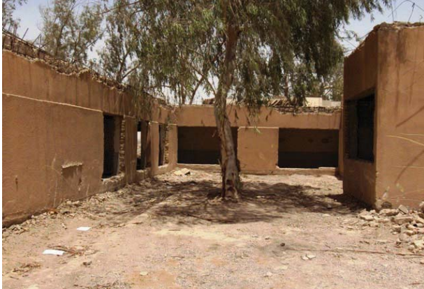
Pre-construction state of building B-230 courtyard, showing the need for extensive renovations. (contractor-provided photo).
