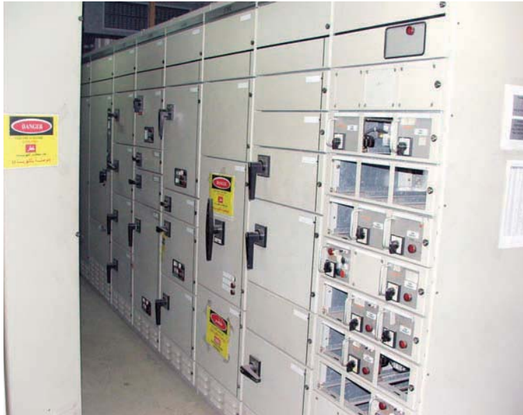
Main control room. Breakers were removed to keep other generators working.
