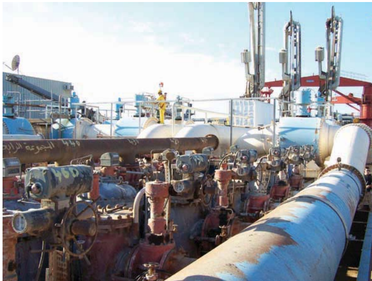
Al Basrah Oil Terminal. Meter work continues to improve the ability of the Iraqi government to monitor oil exports.
