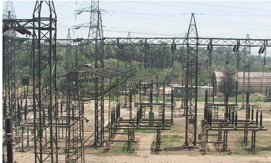
The Iraqi power grid remains very fragile and susceptible to attacks and breakdown.
