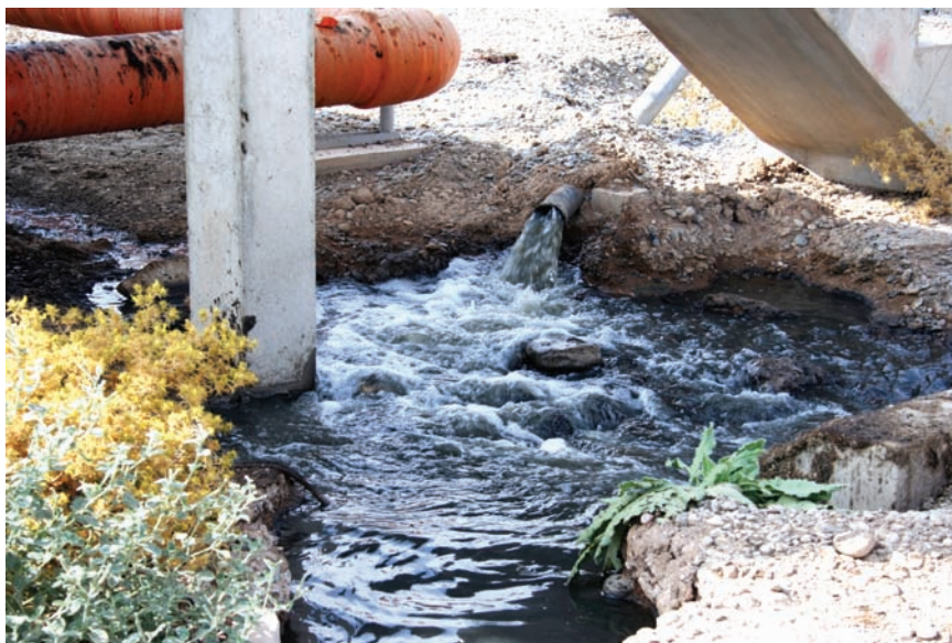
Site Photo 11. Raw sewage pumped offsite through a surface ditch.
