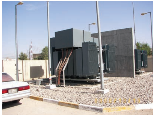
Site Photo 29. Al Serajii 33/11 kV transformer, second assessment.
