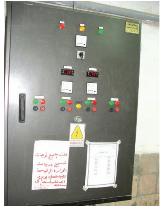
New electrical panel at the Al-Doura Power Plant. This plant has the potential to serve 1.5 million people in Baghdad.
