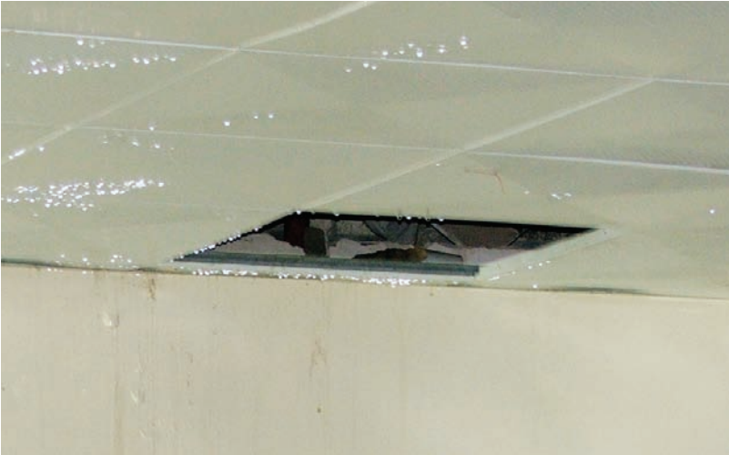
Site Photo 18. Water leaking from ceiling of cadet barracks.
