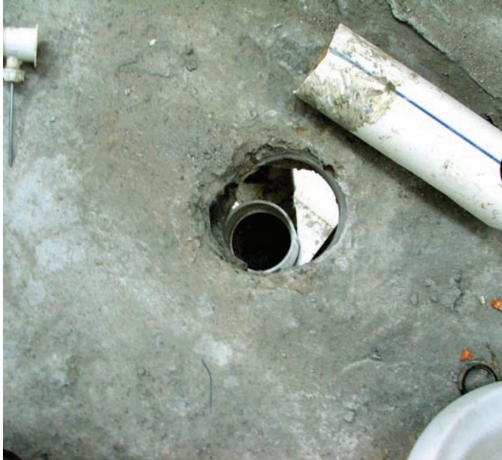
Site Photo 23. Pieces of plumbing pipes in the process of being removed.
