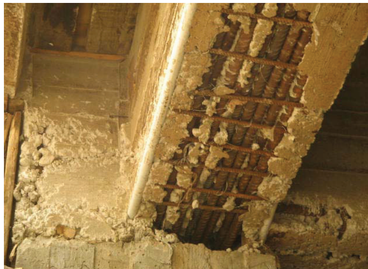
Site Photo 25. Evidence of improperly placed exposed reinforcement bar, PVC conduit, and rust.
