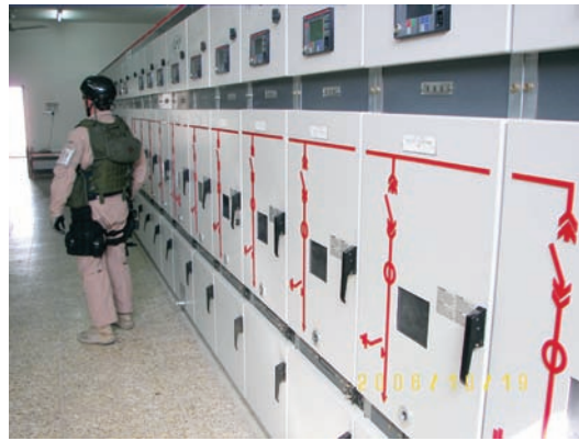
Site Photo 27. Al Hamdan substation distribution: 11 kV switchgear panels at the time of the second assessment.
