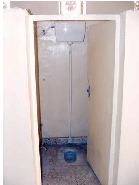
Site Photo 12. Water closet at the 2nd Brigade garrison showing plastic plumbing fixtures.
