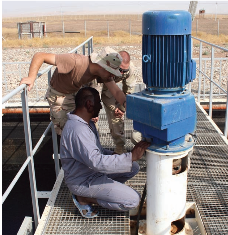
U.S. and Iraqi engineers inspect the broken sweep arm at the Al Kasik Waste Water Treatment Plant.
