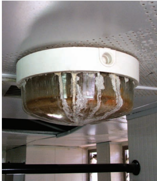
Site Photo 21. Urine-filled ceiling light.
