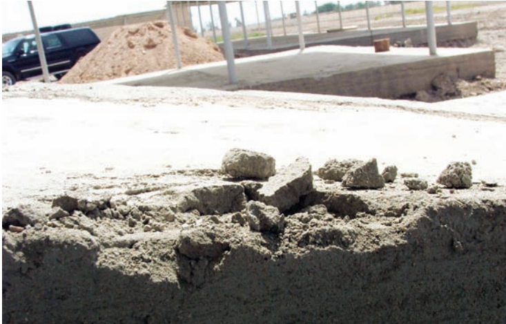
Site Photo 13. Crumbling mortar at the surface of the vehicle ramp.
