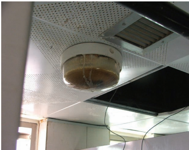
Site Photo 22. Urine-filled ceiling light and hanging wires.
