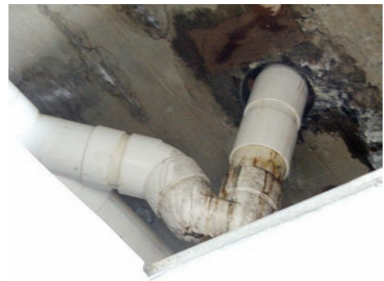
Site Photo 19. Effects of wastewater leaking on plumbing pipes.
