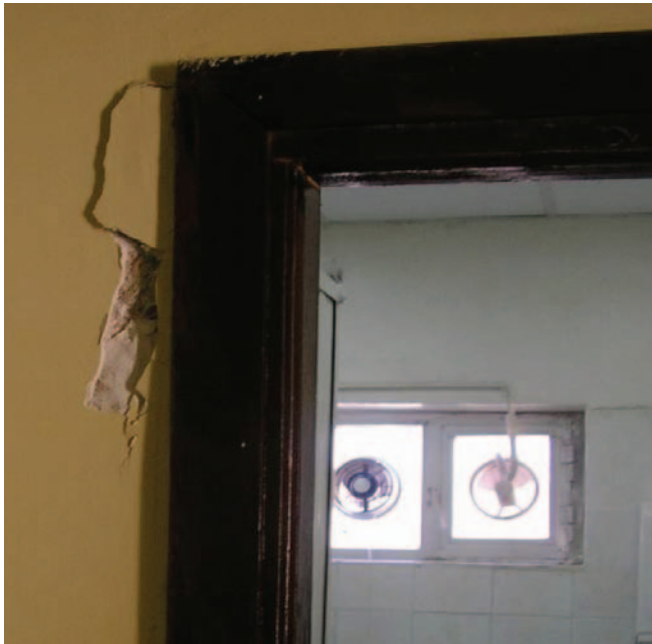
Crack in hallway wall in Instructor Billeting Area (Photo courtesy of contracting officer representative)
