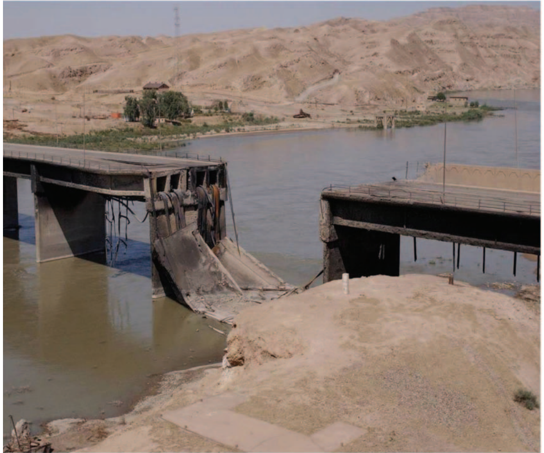
Bomb-damaged bridge crossing the Tigris River at Al Fatah, Iraq
