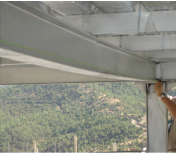
Example of steel I-beam deflection during construction of border forts (Photo courtesy of the Project and Contracting Office)
