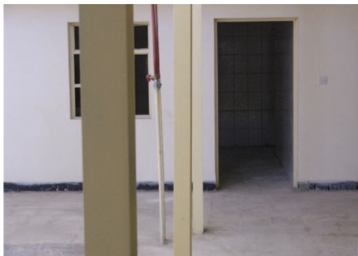
Vertical steel I-beams installed out of proper alignment (not plumb) at border fort
