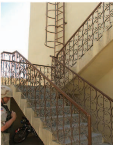
Improper anchoring of staircase railing
