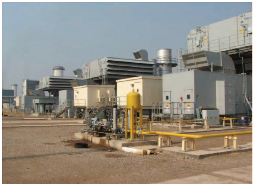
Qudas Power Plant gas turbine generator units
