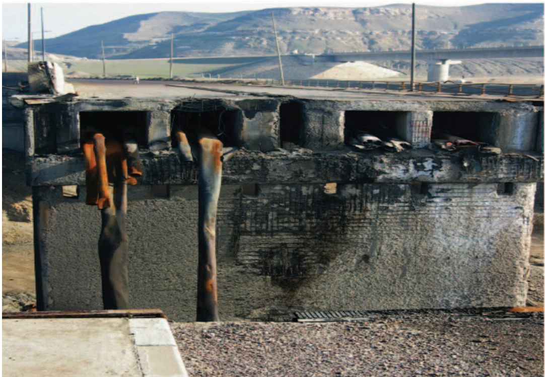
Bridge cross-section showing melted pipes from bomb damage
