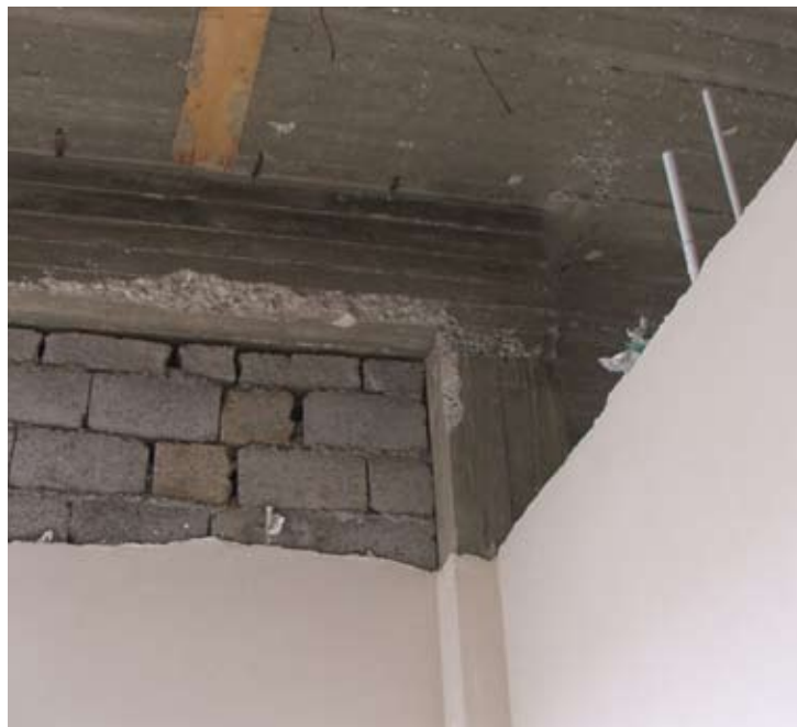
Segregation of load-bearing reinforced concrete ceiling beam
