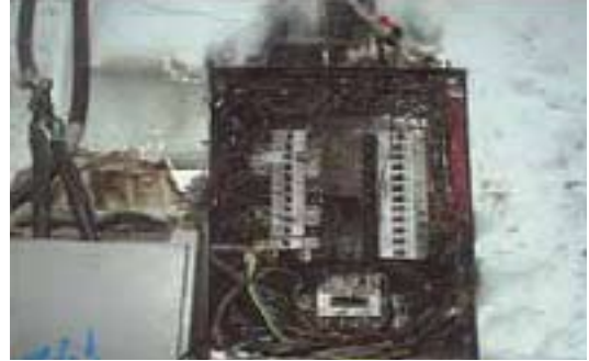
Electrical circuit breaker panel with burn mark
