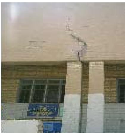
Cracks in school's outer wall
