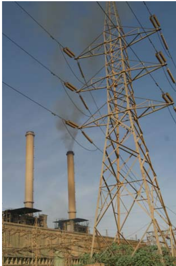
Electricity transmission tower
