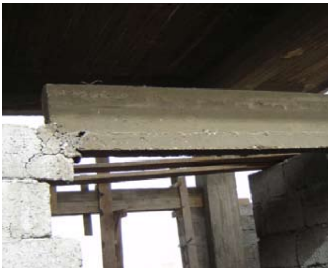
Improperly installed lintel
