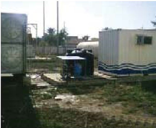
Containerized reverse osmosis unit with storage tanks
