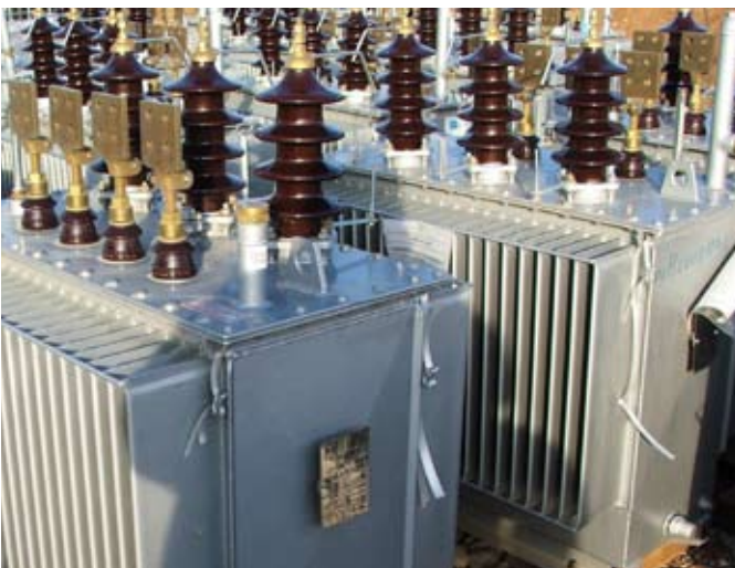
11kV-400V/230V transformers at contractor's storage facility
