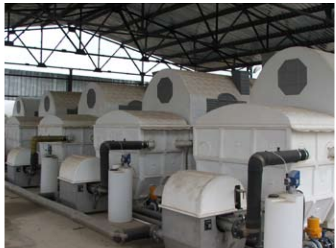
Packaged wastewater treatment plant at Zahko Military Academy
