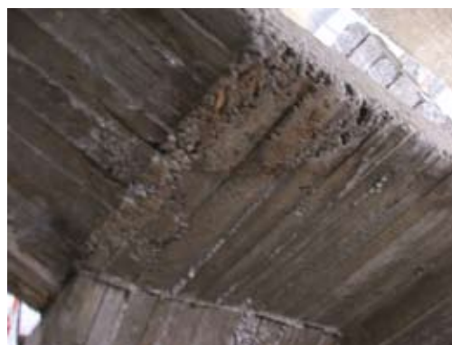
Concrete segregation on underside of reinforced concrete stairwell
