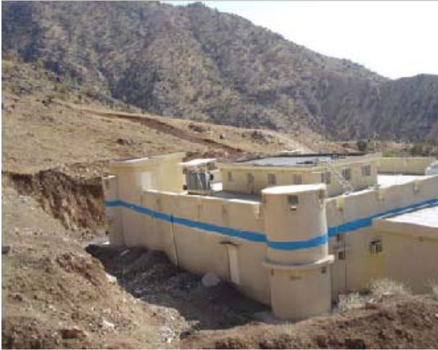
Cut bank with no stabilization at border post
