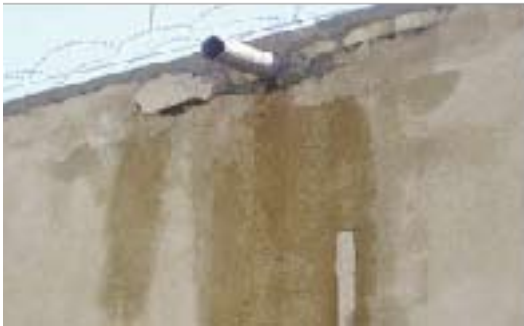
Deteriorating parapet around exterior roof drain
