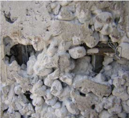
Honeycombing and exposed rebar in concrete—photo provided by U.S. Army Corps of Engineers
