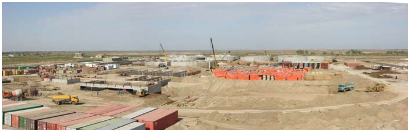
Water treatment plant at Nassriya
