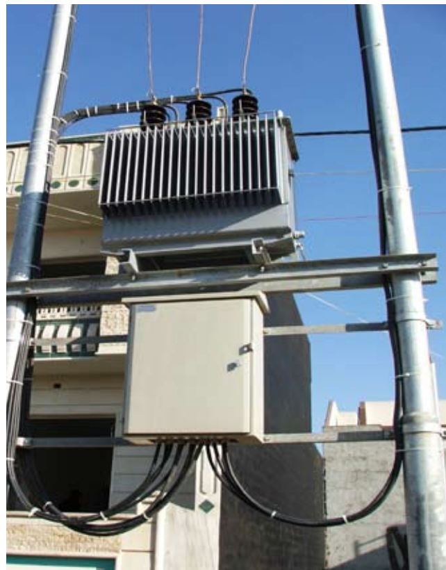
Transformer and low voltage electrical distribution panel
