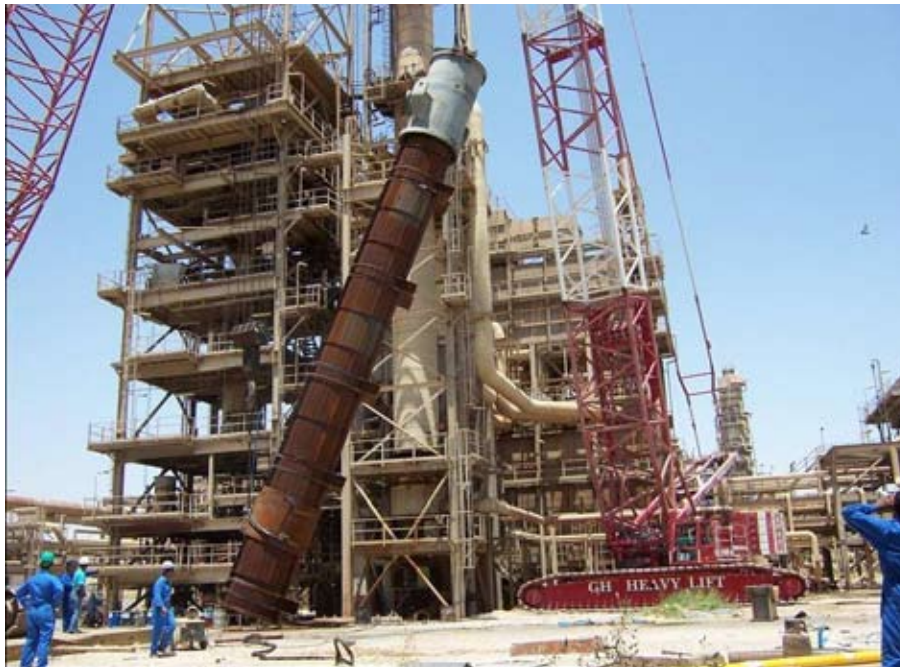
Liquid petroleum gas plant at Khor Zubair
