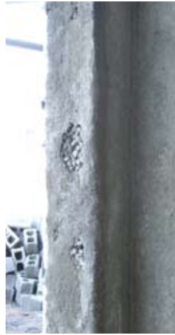
Honeycombing after surface coating
