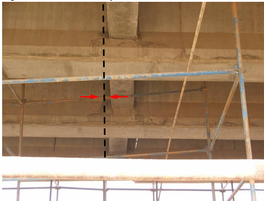
Site Photo 13. Misaligned diaphragms
