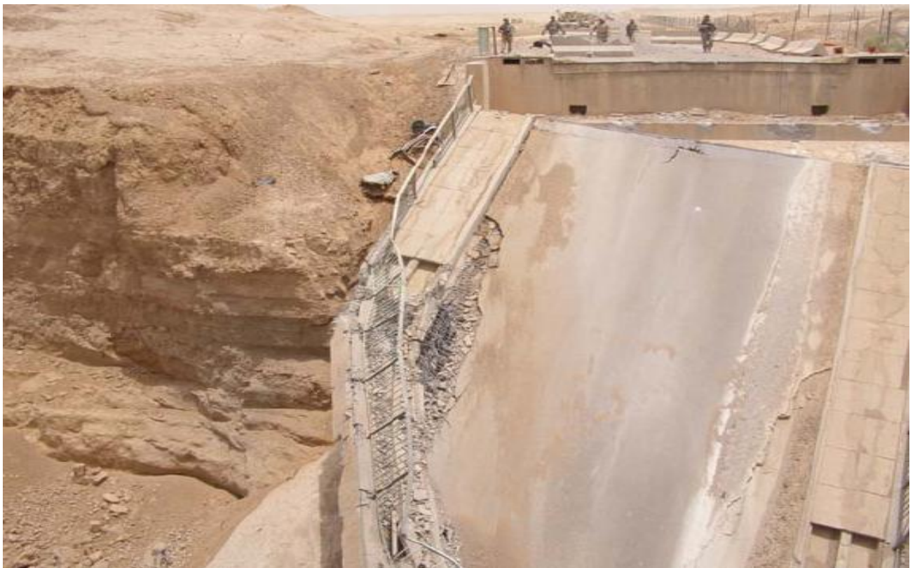
Site Photo 4. Mugarrah Canal Bridge with VBIED damage to Span No. 1 (Courtesy of GRC)
