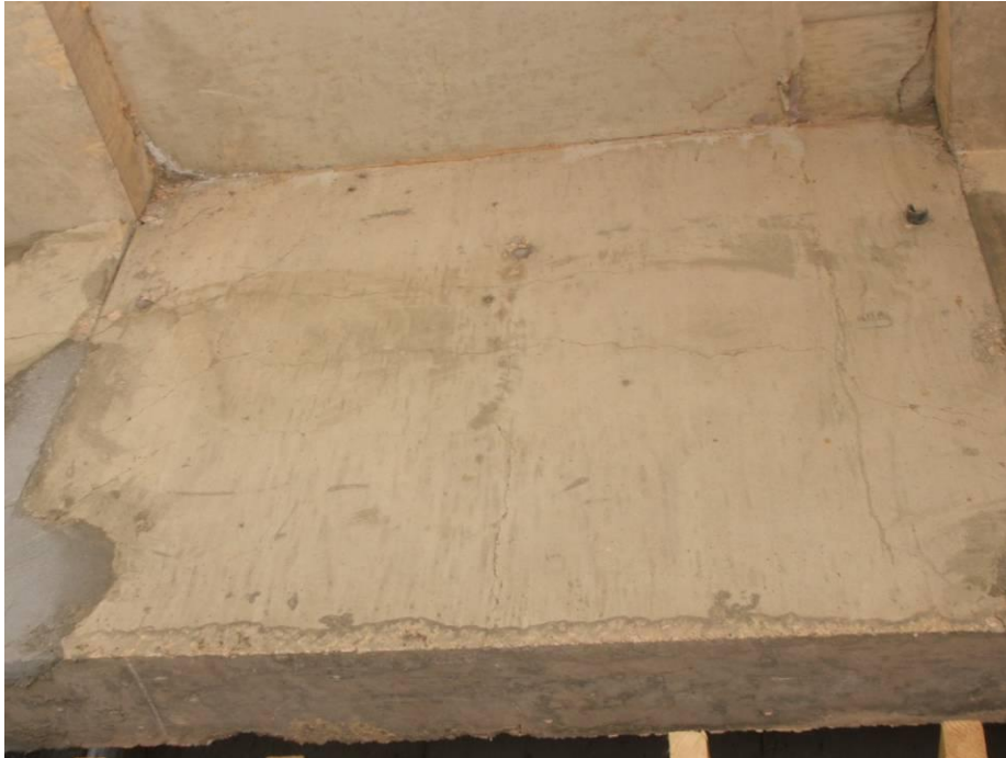
Site Photo 14. Existing damaged diaphragm at Bent No. 1
