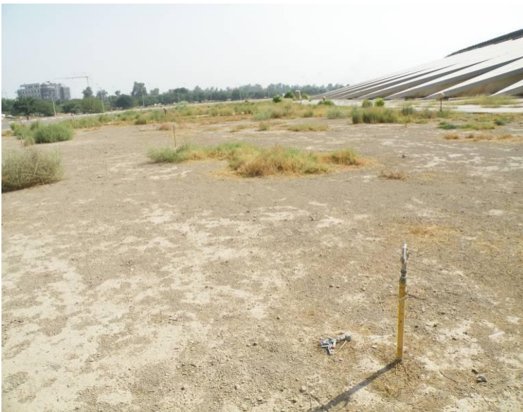
Site Photo 10. Sprinkler heads
