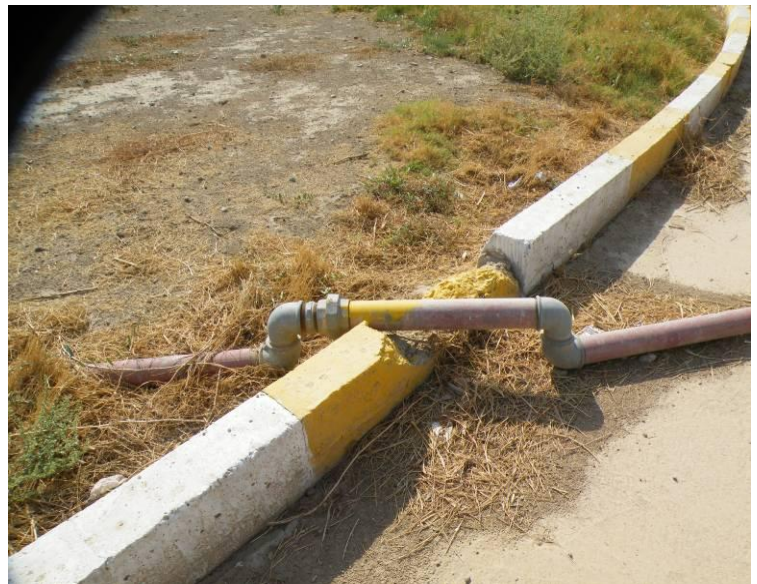
Site Photo 11. Honor Unit representatives stated the contractor used existing pipes
