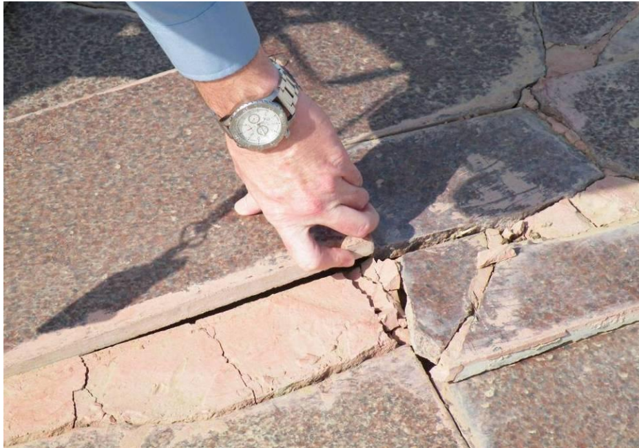
Site Photo 6. Cracked and raised concrete tiles
