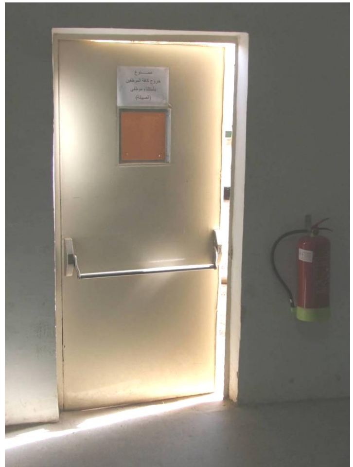
Site Photo 10. Door unable to fully swing open
