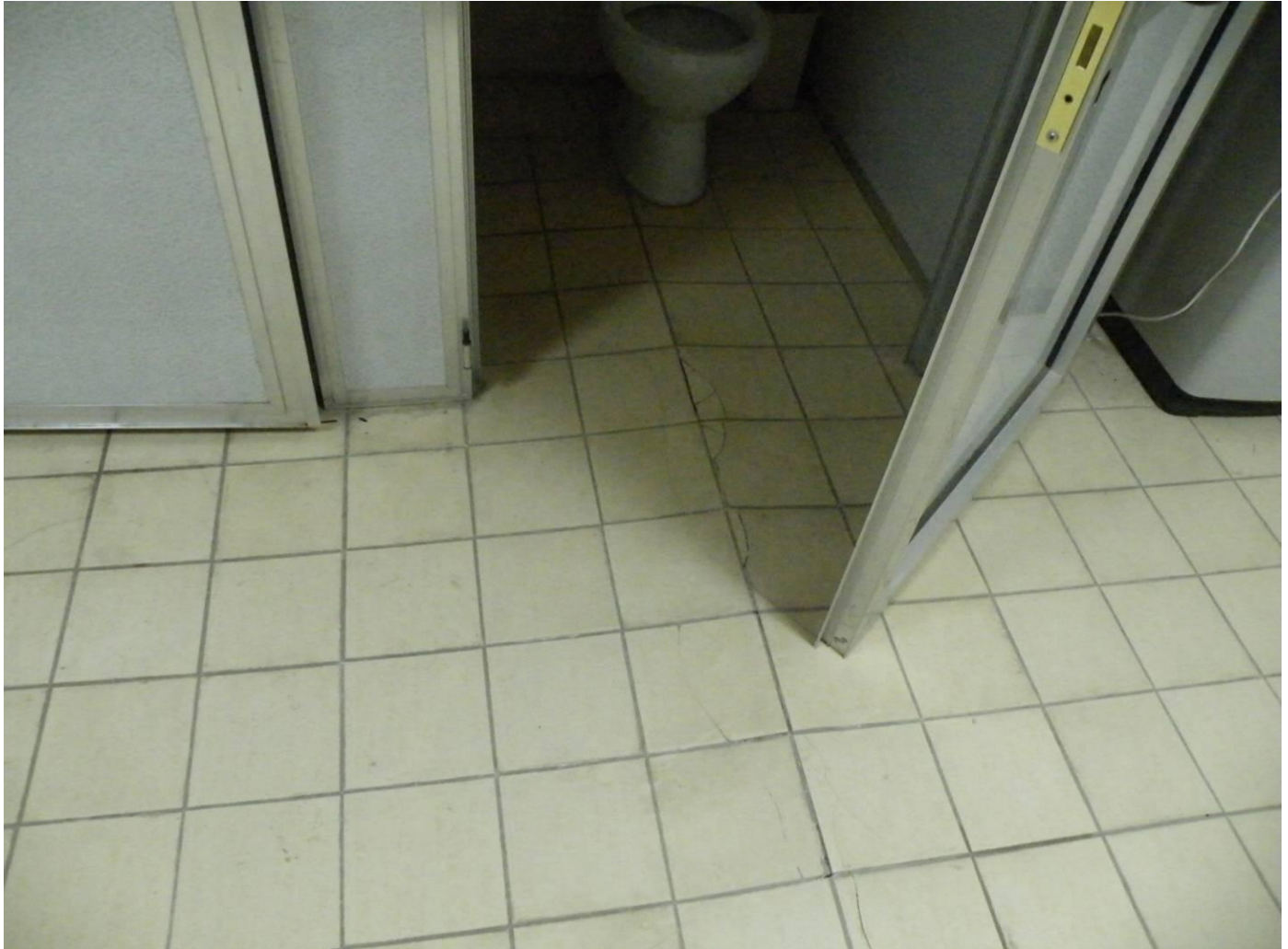
Site Photo 8. Example of tile cracking and buckling inside SDSF latrine
