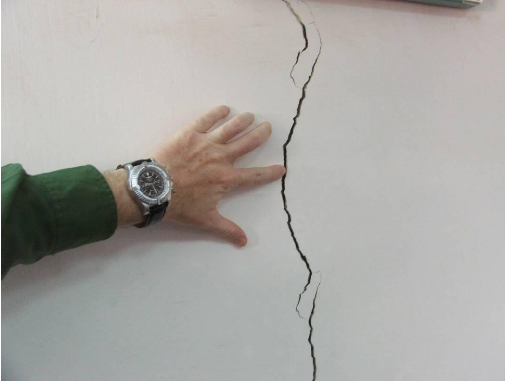
Site Photo 14. Example of cracking of interior wall
