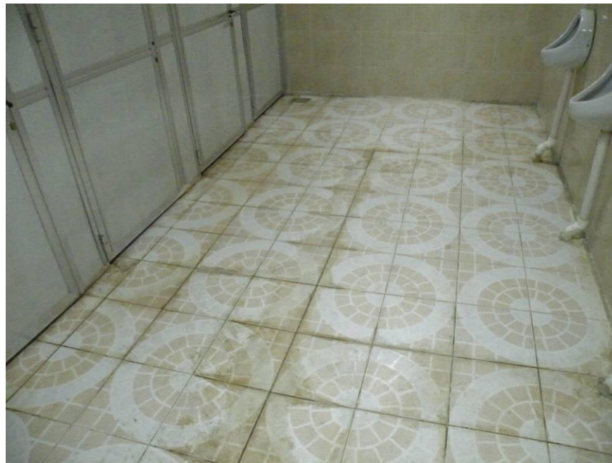
Site Photo 15. Contractor replaced previously cracked and buckling floor tiles (See Site Photo 8 for original condition of bathroom floor.)
