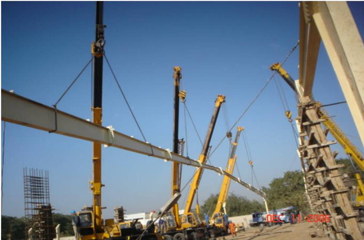
Site Photo 1. Initial construction of the steel columns prior to the structural failure (Courtesy of GRC)
