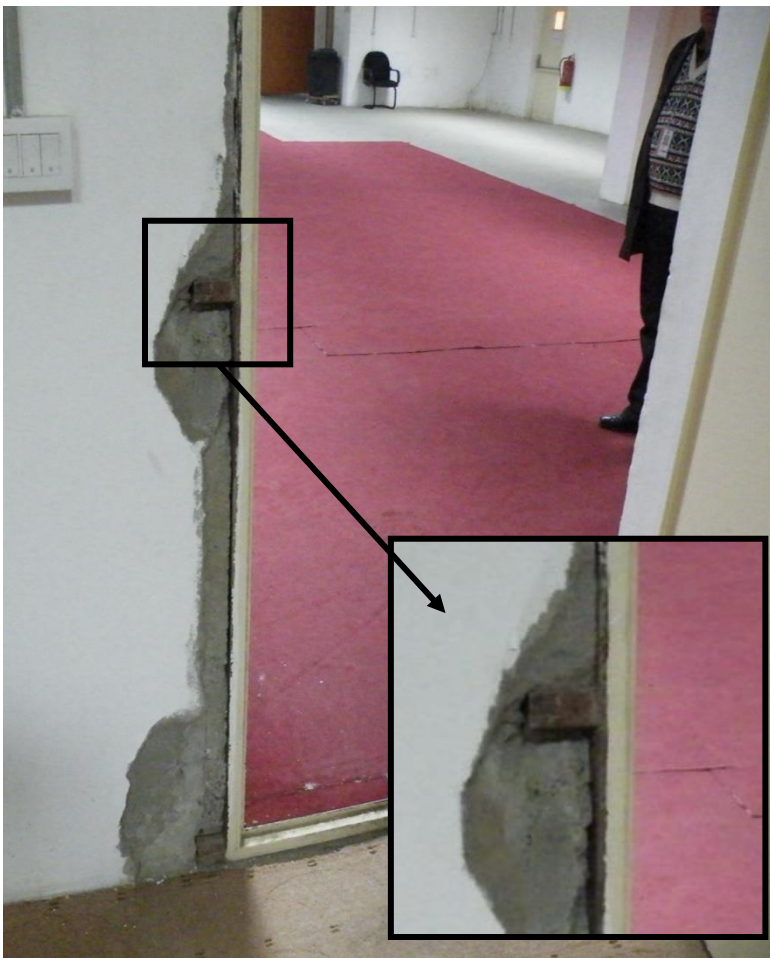
Site Photo 9. Interior door damage
