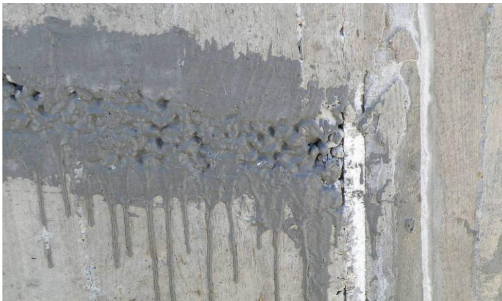
Site Photo 10. Attempted repair of honeycombing utilizing low viscosity epoxy
