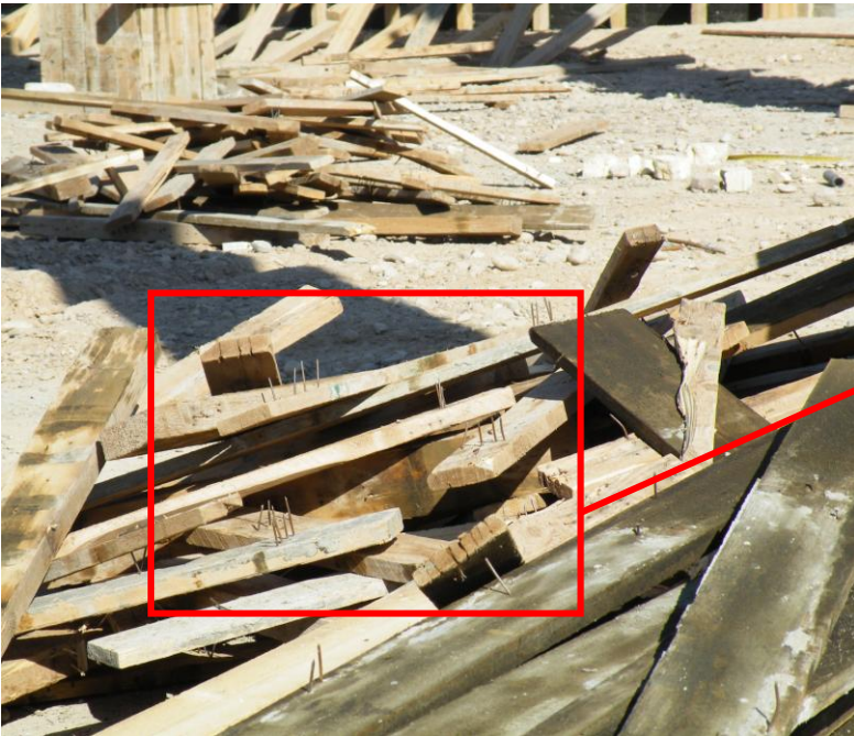
Site Photo 21. Example of protruding nails
