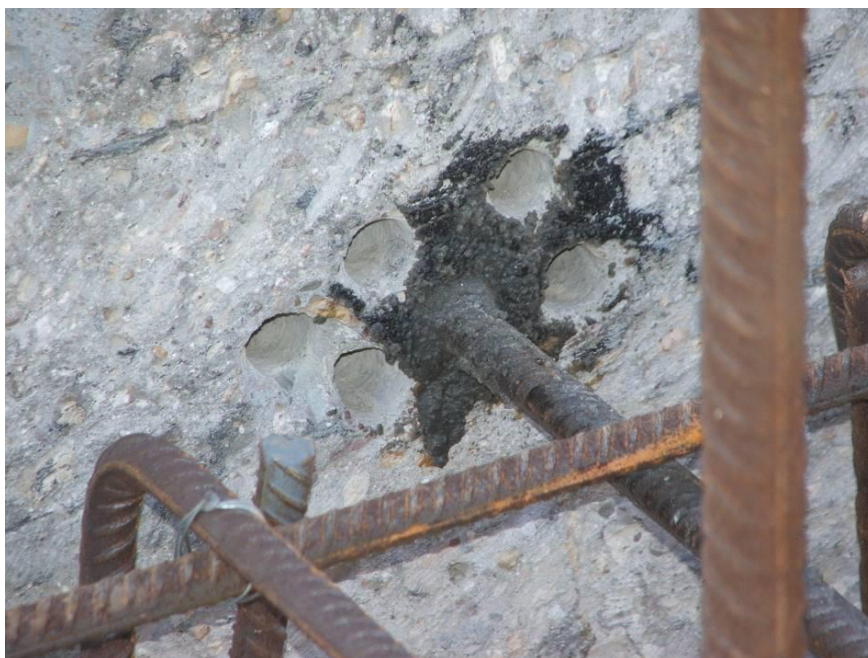
Site Photo 13. Multiple holes surrounding epoxy anchored dowel
