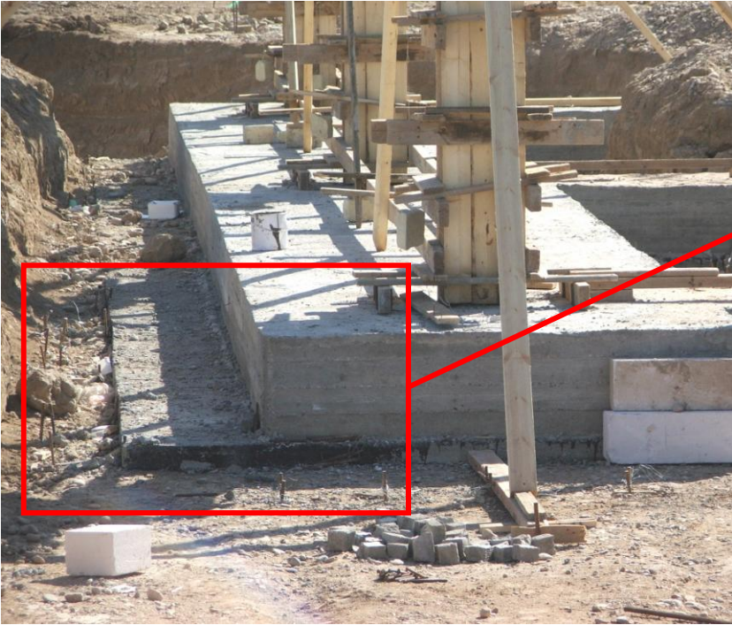
Site Photo 19. Examples of protruding reinforcement bar
