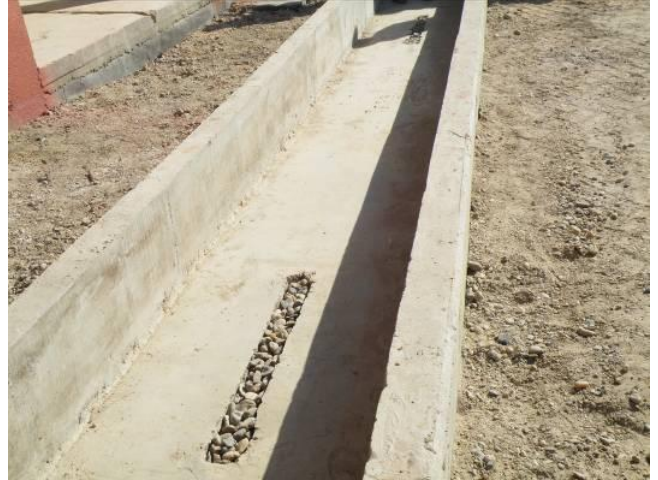
Site Photo 8. Cable trench interior
