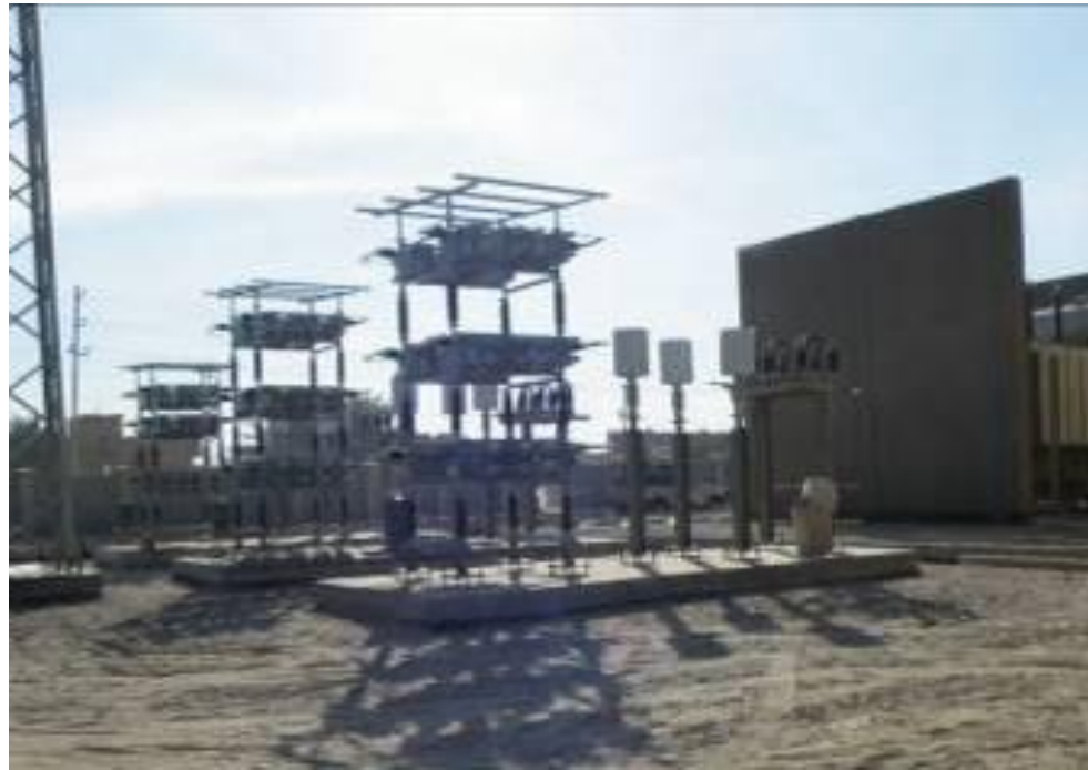
Site Photo 14. Capacitor banks
