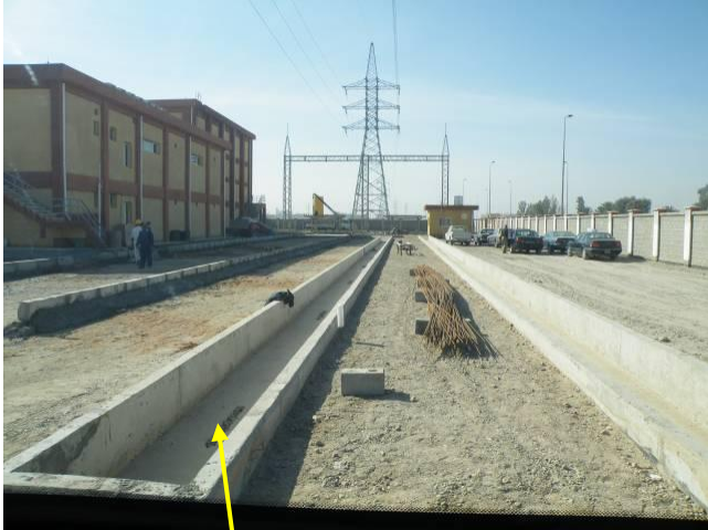
Site Photo 7. Cable trenches
