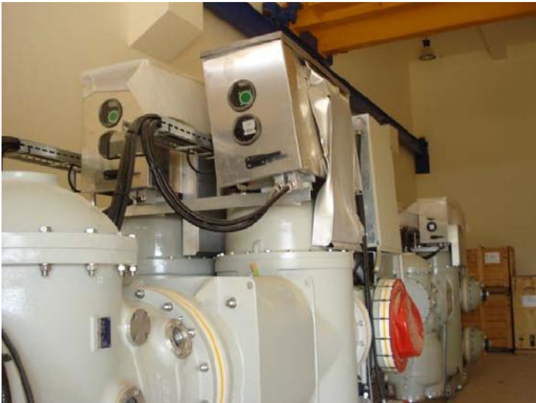
Site Photo 19. GIS E05 and E06 (Courtesy of USACE)
