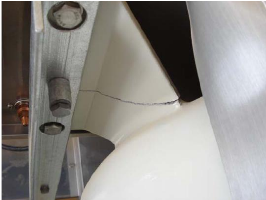
Site Photo 20. Cracked GIS E05 and E06 (Courtesy of USACE)
