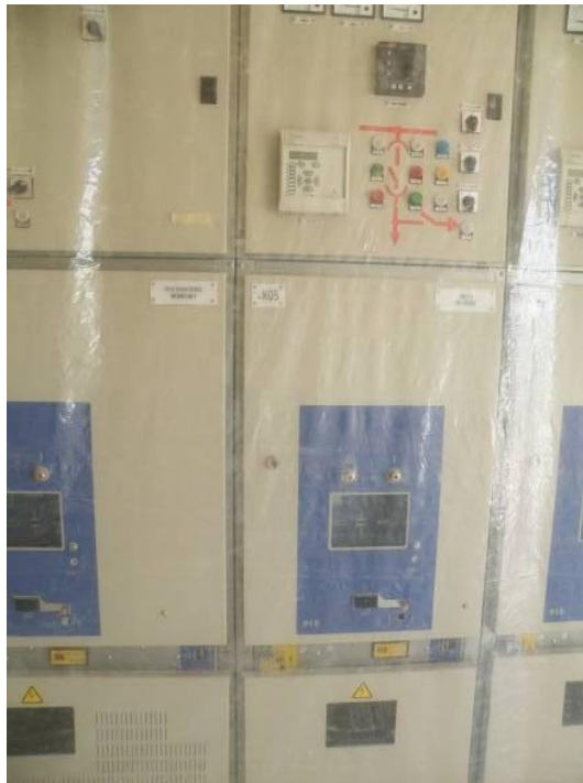
Site Photo 13. Electric metering equipment
