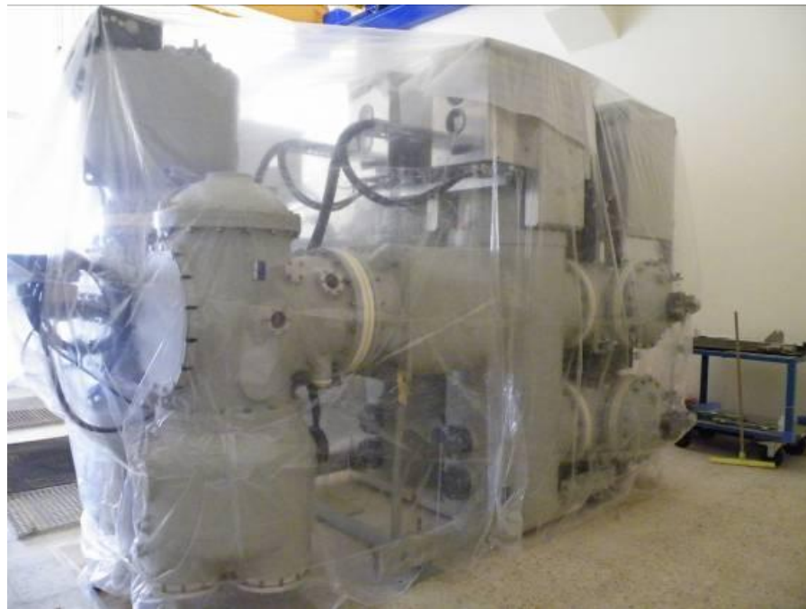
Site Photo 11. Gas insulated switch
