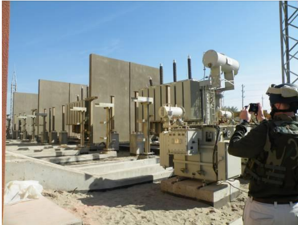
Site Photo 16. Transformer bays
