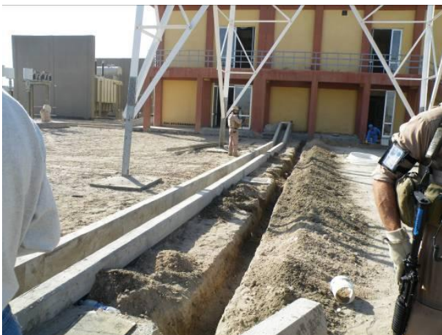
Site Photo 9. Cable trench entering building
