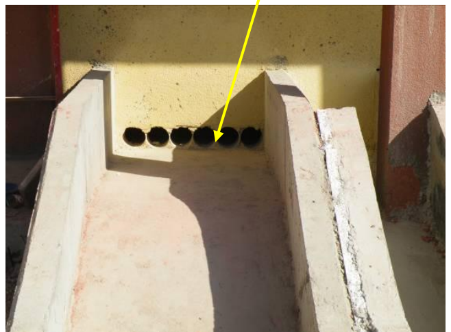
Site Photo 10. Entrances for cables
