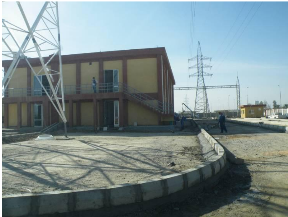
Site Photo 18. Non-compacted road
