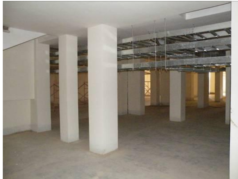
Site Photo 6. Interior substation ground floor columns & cable trays
